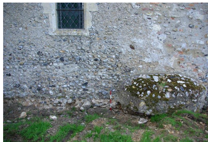
Plate 6: Base of chancel wall and rood turret remains prior to repair, looking S, 0.5m scale
