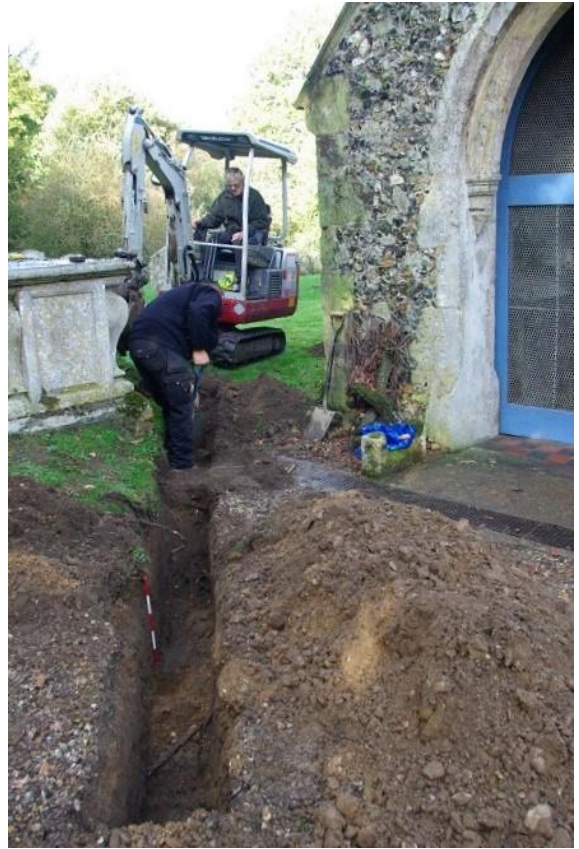
Plate 5: Trench S of porch, existing electric cable visible, looking NW, 0.5m scale
