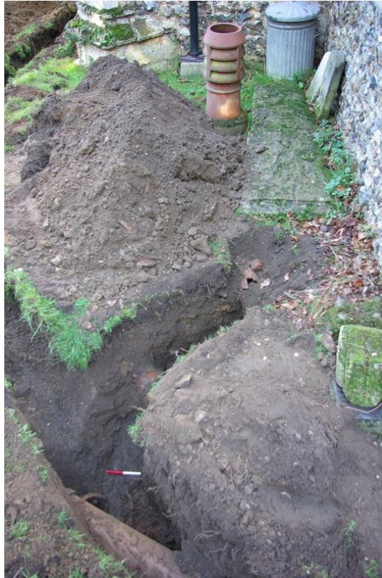
Plate 2: Trench W of porch; burial [2] visible below drain pipe, looking N, 0.5m scale
