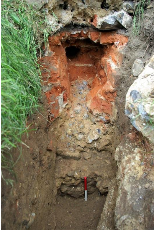
Plate 6: N aisle stepped footing [9], brick footing [4] partly removed, looking S, 0.5m and 0.2m scales
