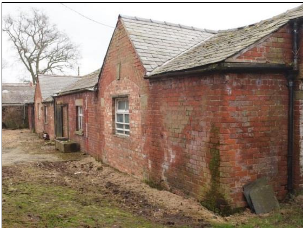
Plate 35: West end of north elevation showing western gable and blocked cart doorway
