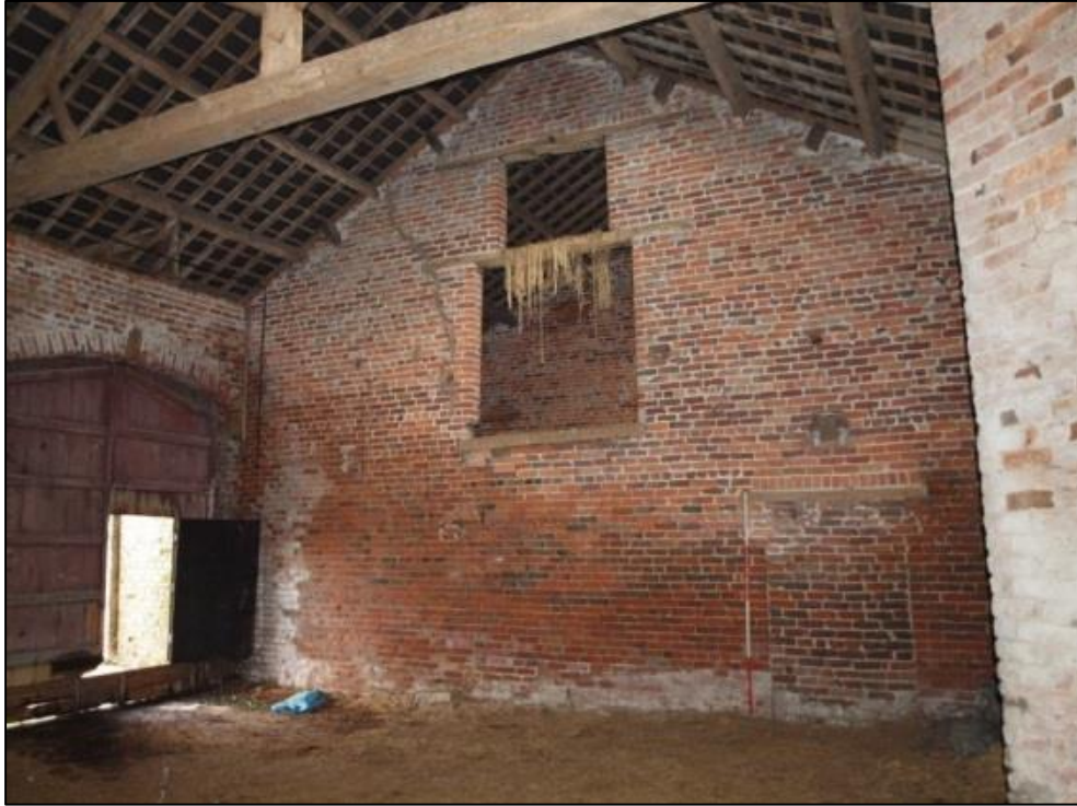
Plate 22: North internal wall showing blocked doorway and pitching windows to first floor
