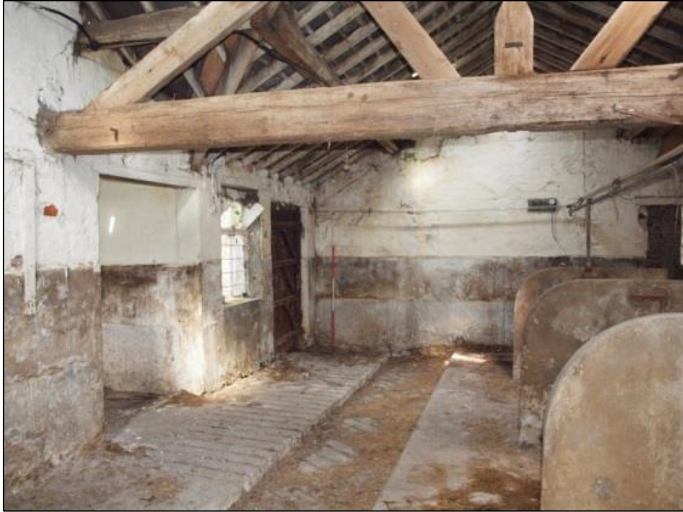
Plate 42: As above, showing inserted doorway to barn (far right) and external doorway (left)
