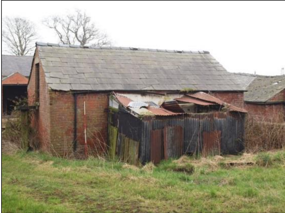
Plate 53: West (rear) elevation with dilapidated lean-to.
