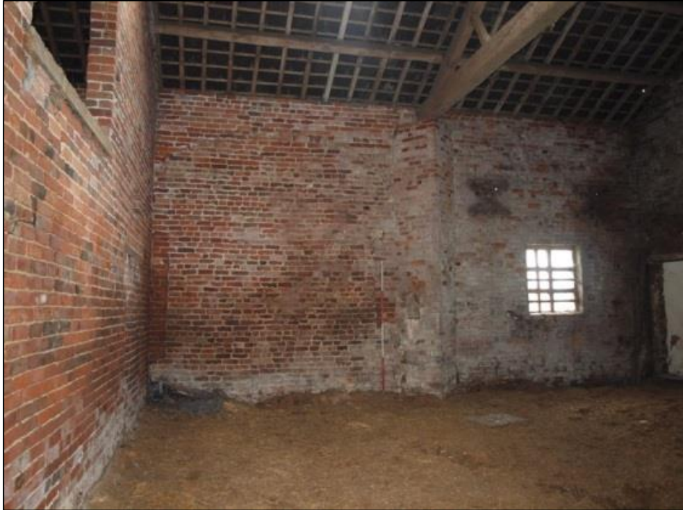
Plate 20 Interior of barn showing blocked barn door
