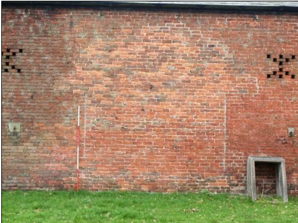
Plate 15: Blocked barn door in east elevation
