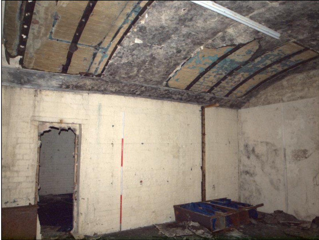
Plate 45: Second unit showing inserted doorway, rear wall and bricks of the vaulted roof
