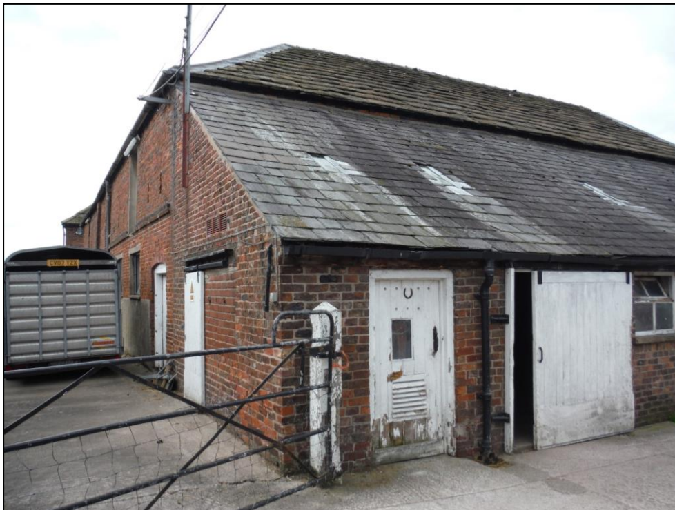
Plate 6a: As above before the scaffolding and general deterioration
