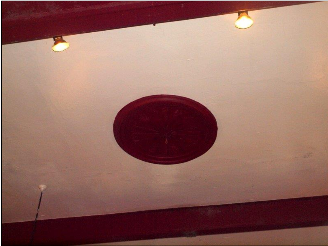
Plate 27: Plaster ceiling rose at north end of church
