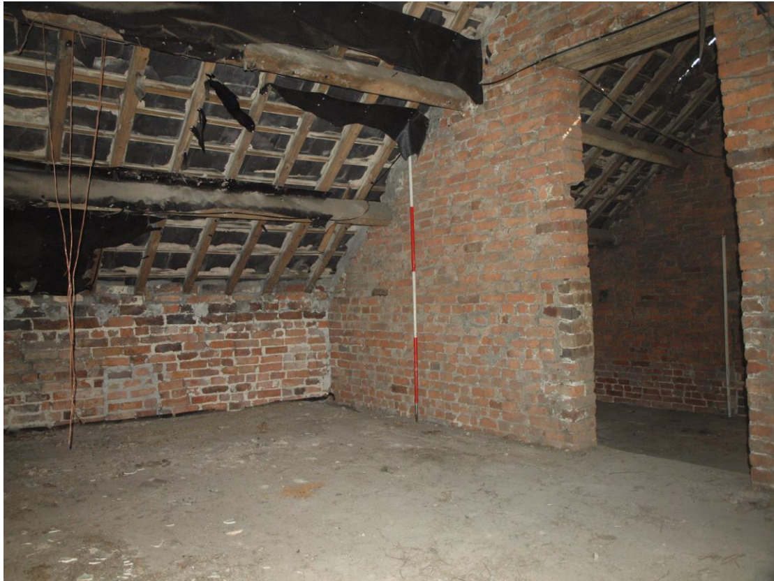
Plate 25: Doorway to room 2. Note the notch in the jamb where a former lintel has been removed, suggesting a lower door with opening over.
