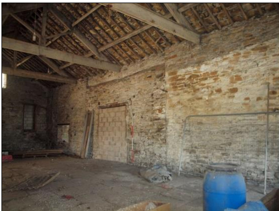
Plate 16: Barn interior showing other side of blocked loading door and barn door
