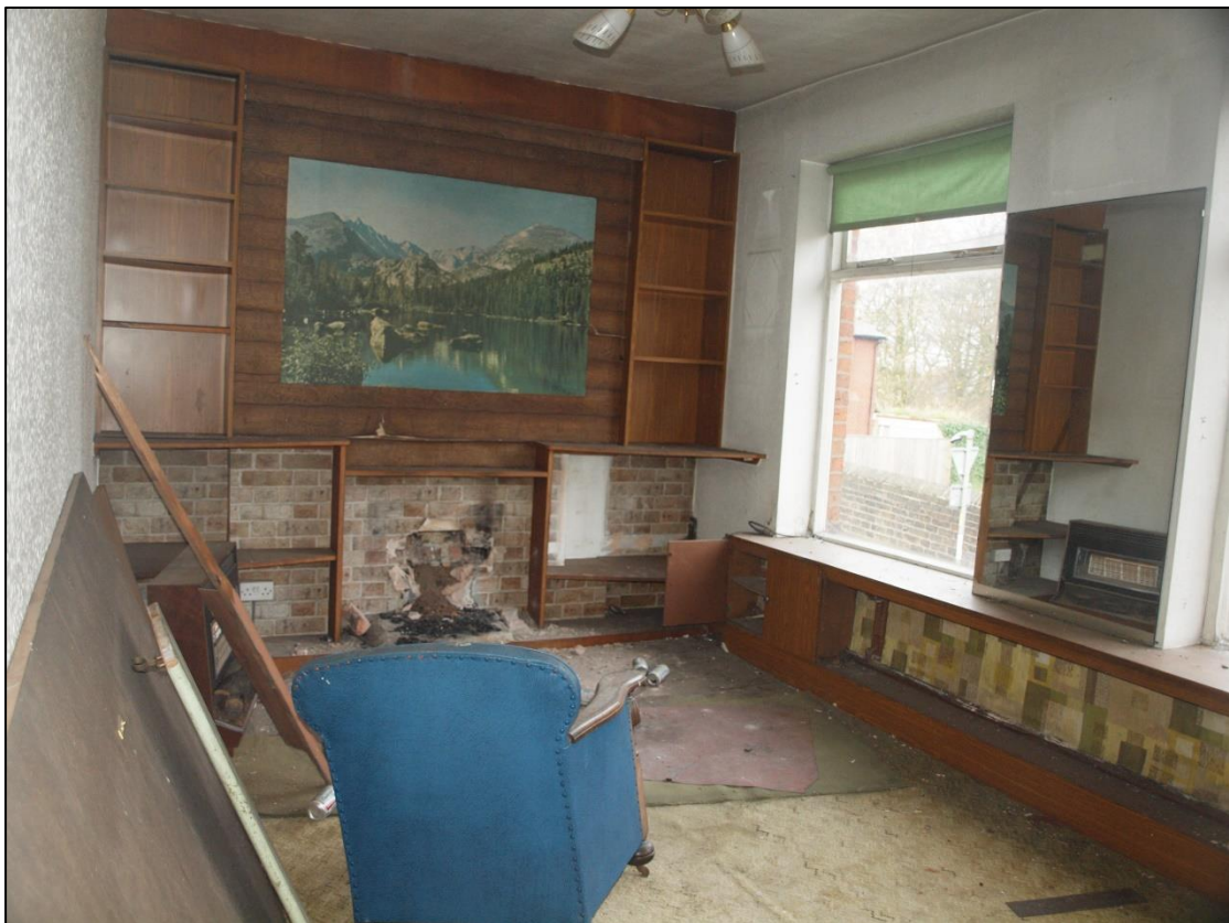
Plate 58: Dilapidated lath and plaster ceiling in first floor of number 5
