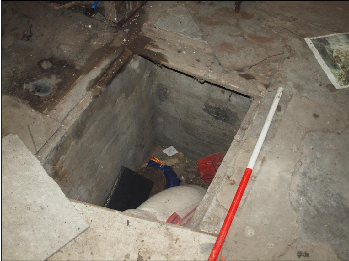
Plate 41: Concrete hole in floor of 7 - 9
