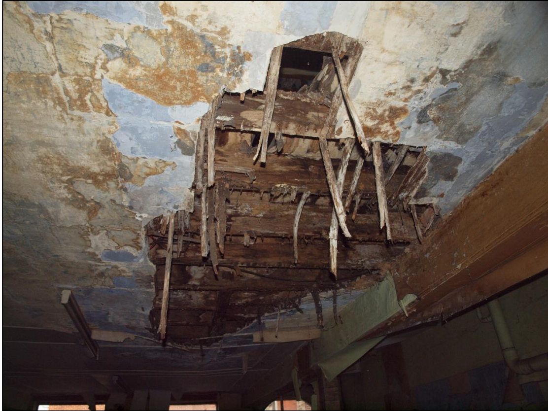
Plate 21: Dilapidated lath and plaster ceiling of number 5
