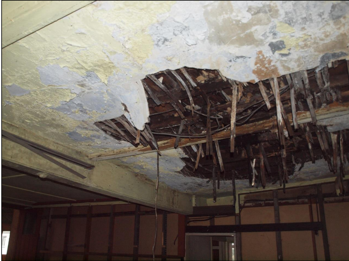
Plate 57: Dilapidated lath and plaster ceiling in first floor of number 5
