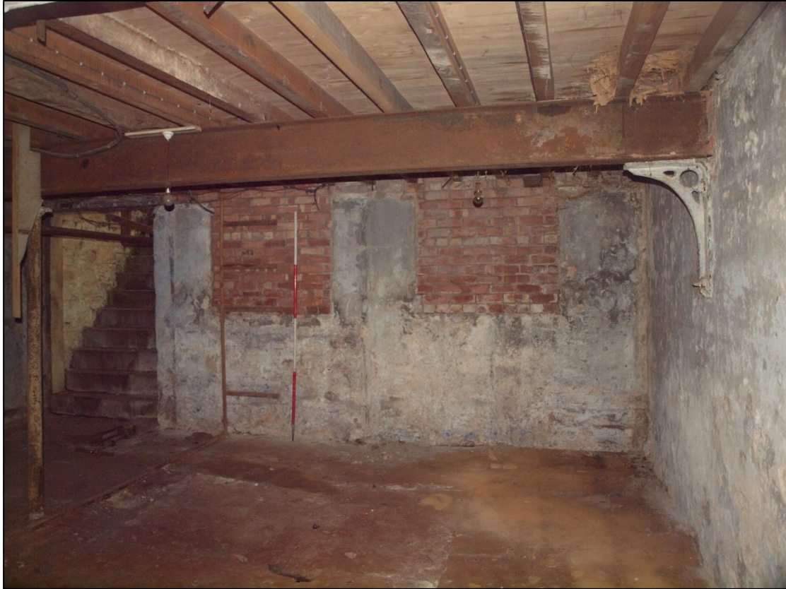
Plate 51: Blocked cellar lights in rear wall
