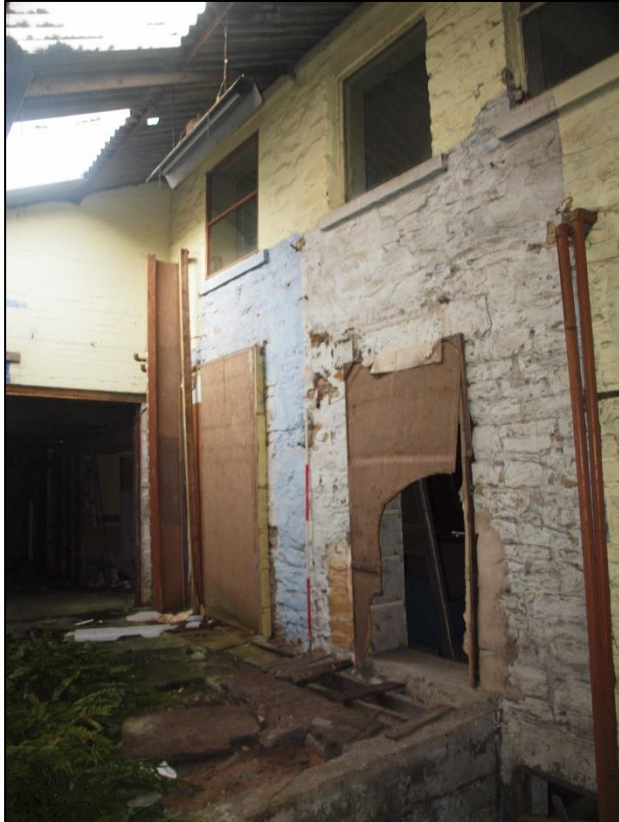
Plate 29: Former rear wall of number 5 showing blocked inserted doorways
