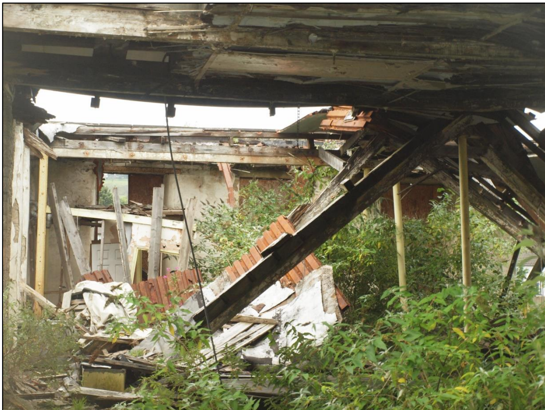
Plate 52: Detail of collapsed roof
