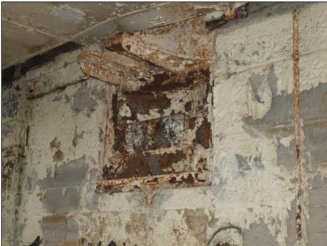
Plate 50: Detail of blocked transmission window
