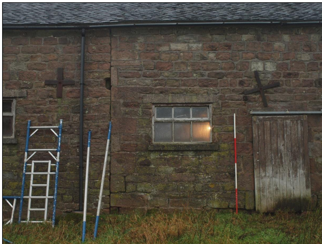
Plate 28: Straight joint between bays 3 and 4
