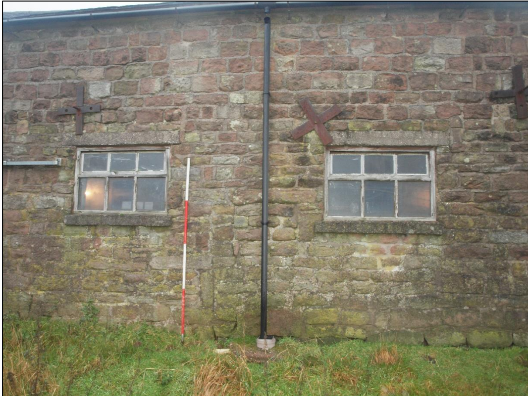
Plate 25: Blocked doorway to bay 2
