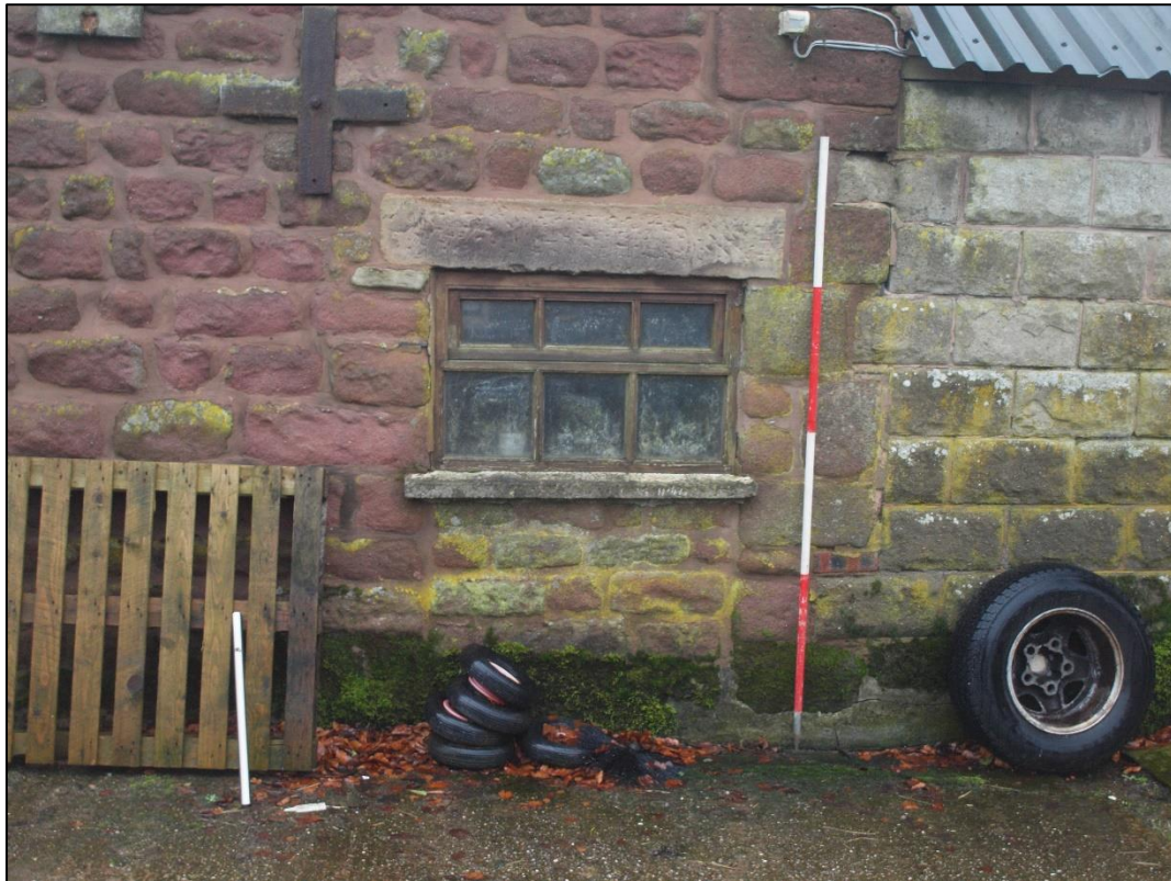
Plate 17: As above showing rough joint to modern extension
