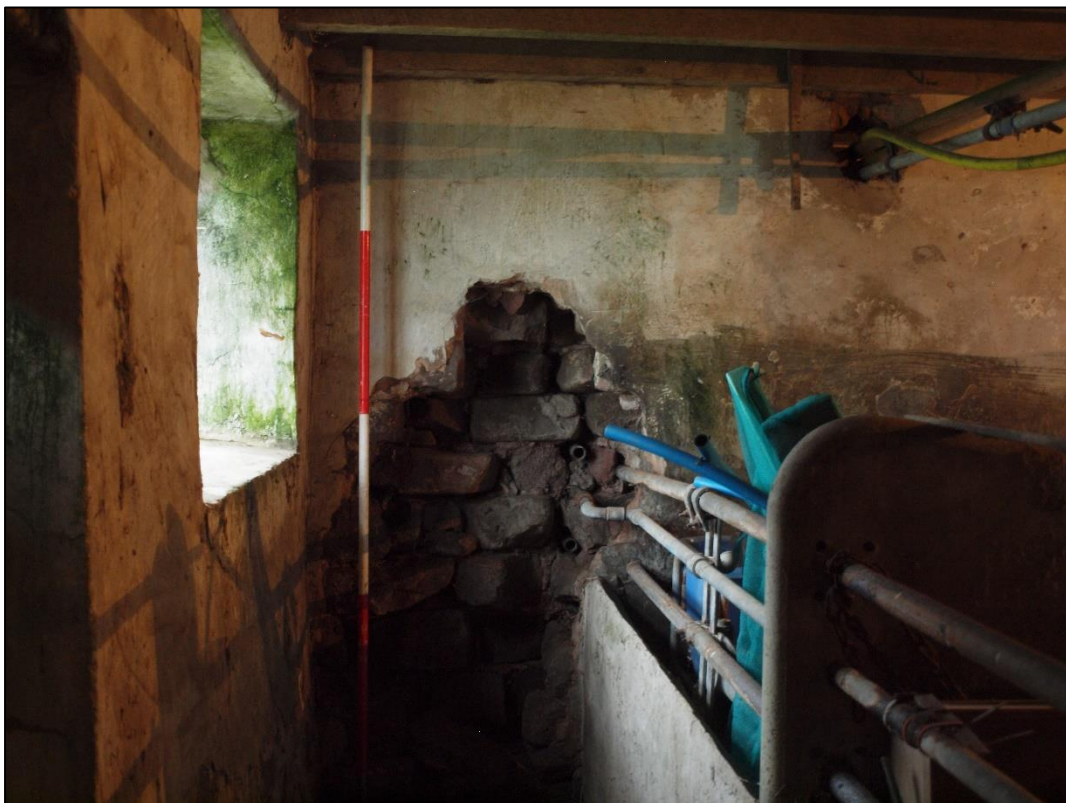
Plate 44: Detail of partially removed wall in cross wall where doorway would be expected
