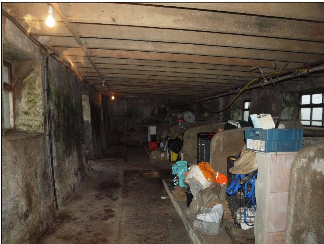
Plate 34: General shot of ground floor interior showing manure passage and concrete boskins
