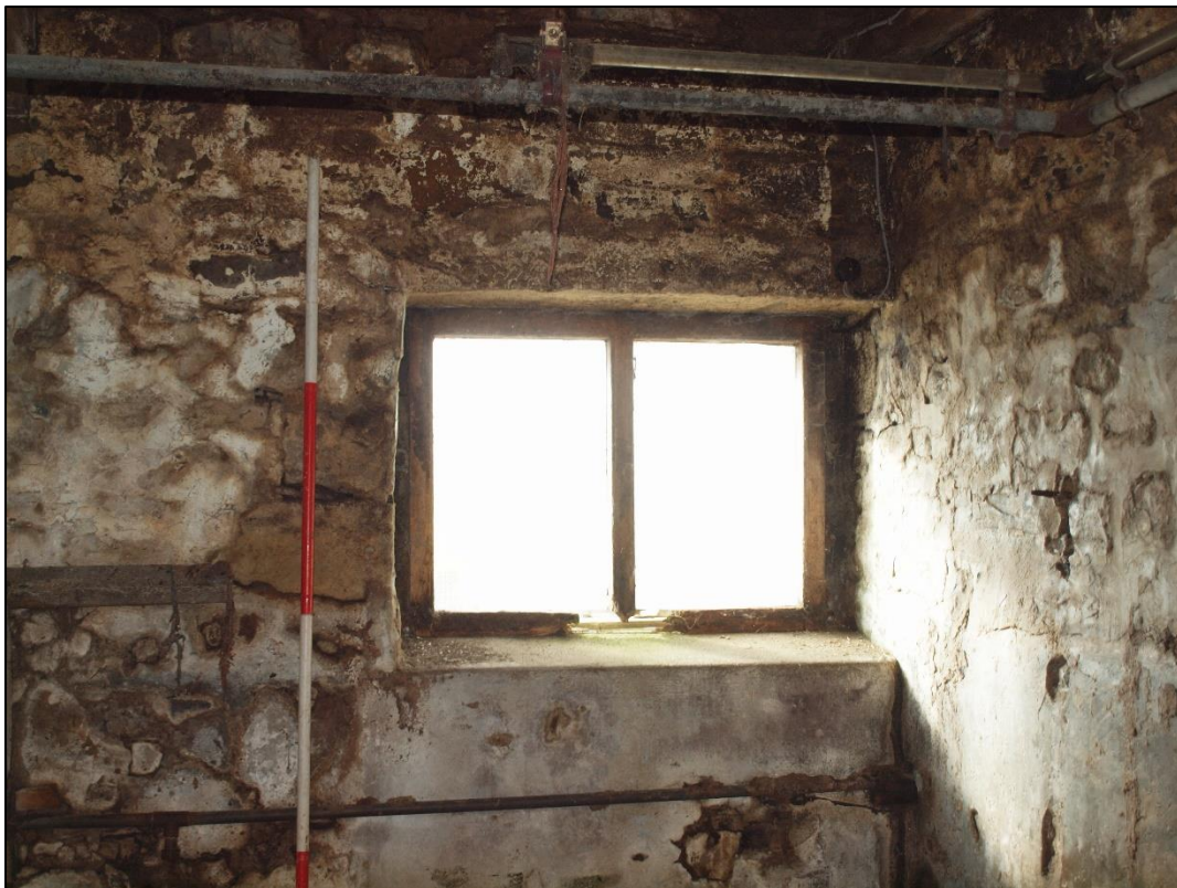
Plate 24: Detail of window with stone lintel in west end of south elevation
