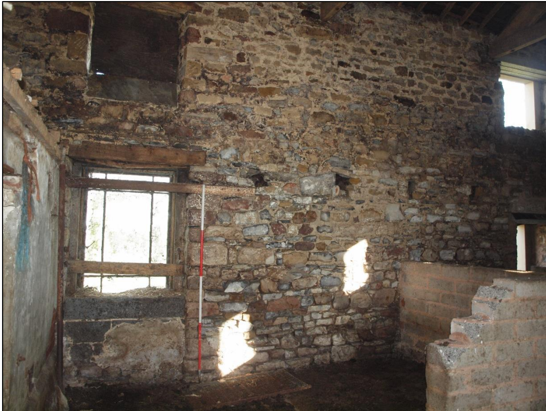
Plate 27: Central area showing former threshing door and visible joist holes in north wall
