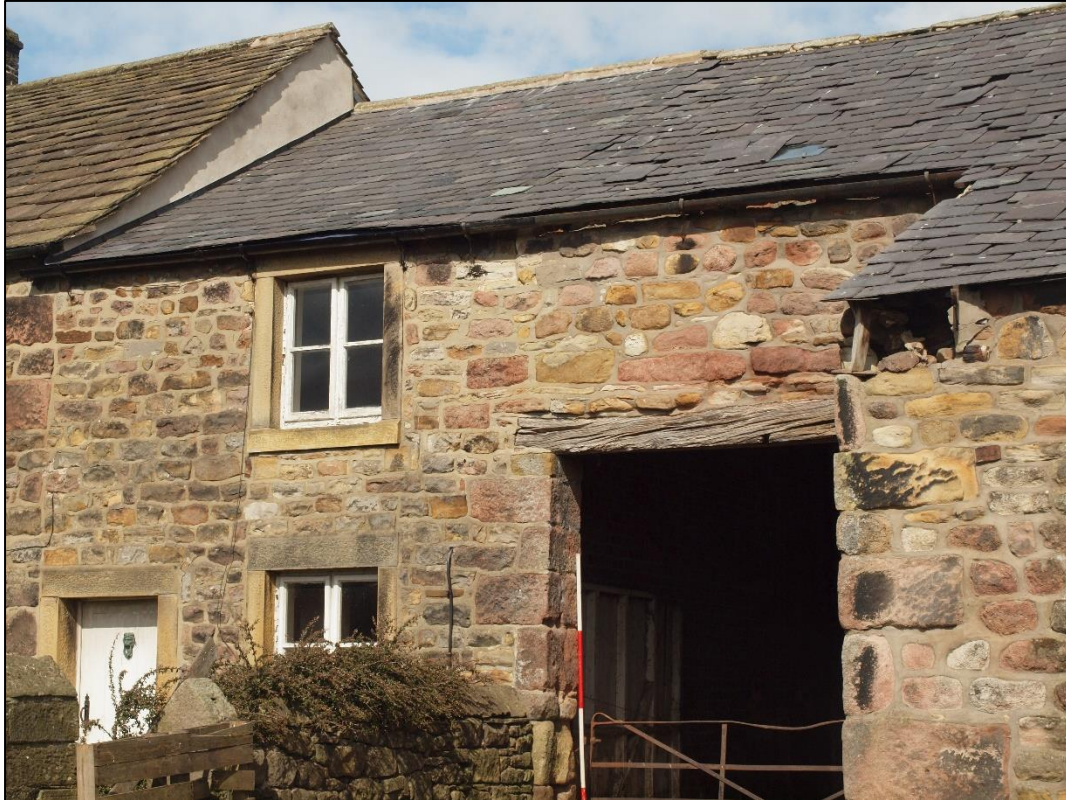
Plate 19: Shot showing converted bay of barn. Note the straight joint between the house and barn (far left)
