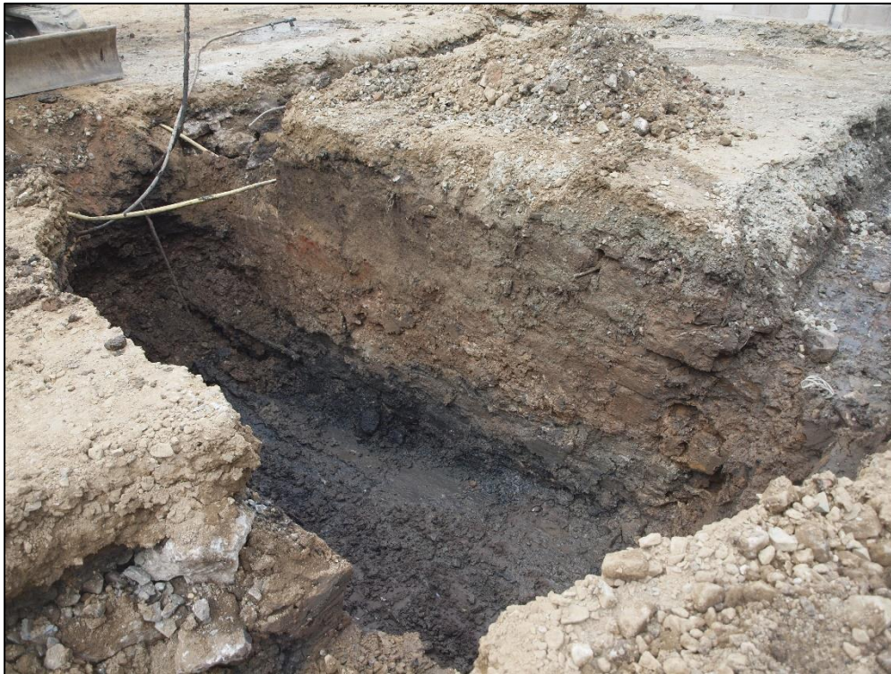
Plate 19: Central trench after collapse of northern side showing flags (05) at base below grey clay (04)
