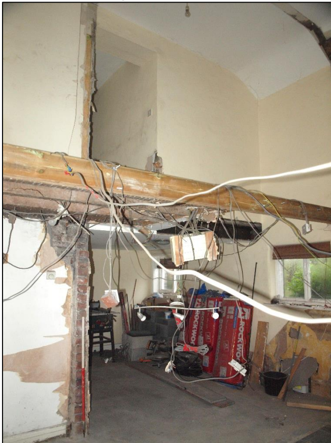
Plate 50: Extension looking towards main house showing removed ceiling
