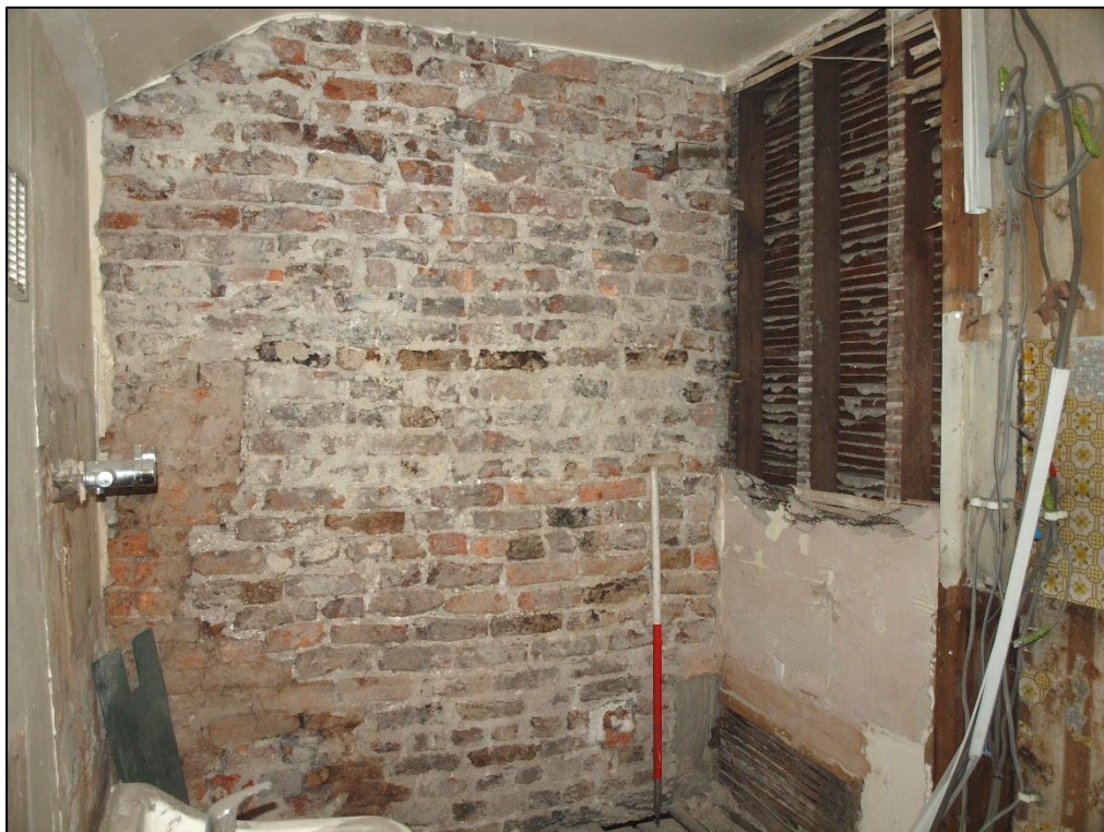
Plate 72: As above showing blocked opening in brickwork and lath and plaster wall
