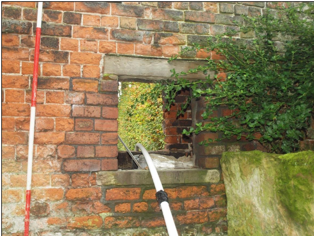
Plate 10: Detail of inserted window shown above
