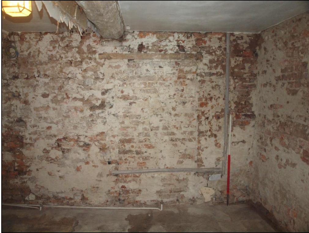
Plate 41: Detail of blocked door to living room
