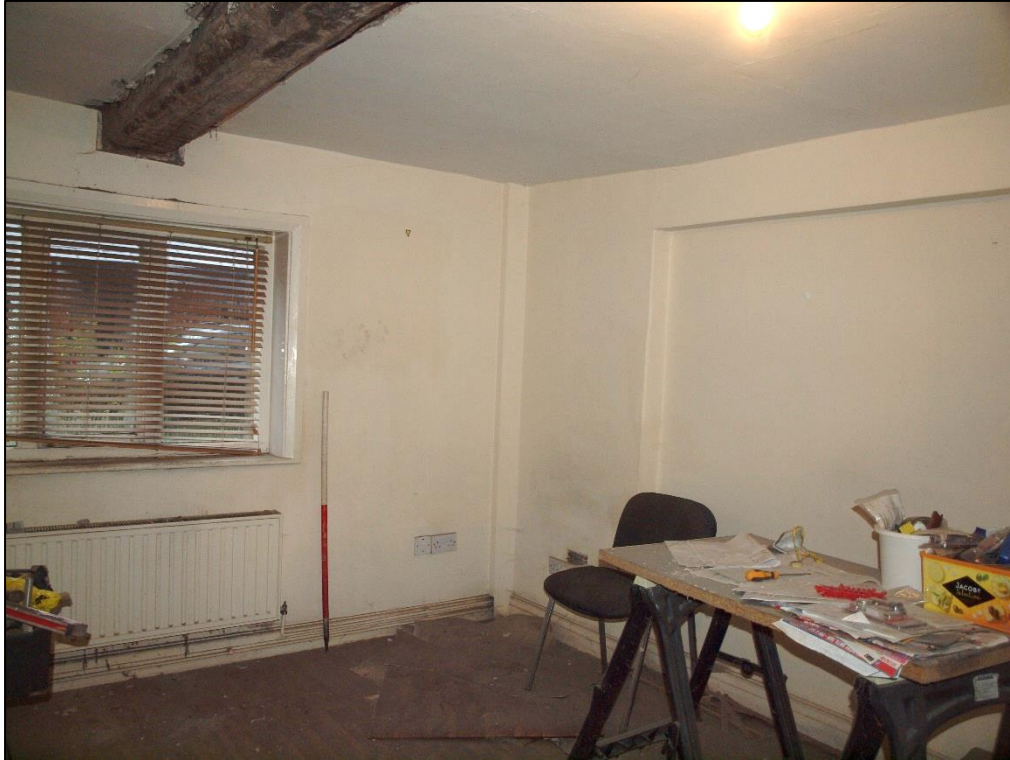
Plate 51: Room to south corner of main house showing blocked opening to right
