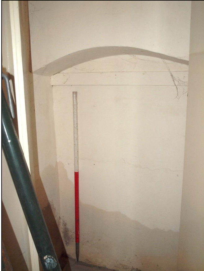
Plate 55: Arch of chimney breast moving to the north of the fireplace
