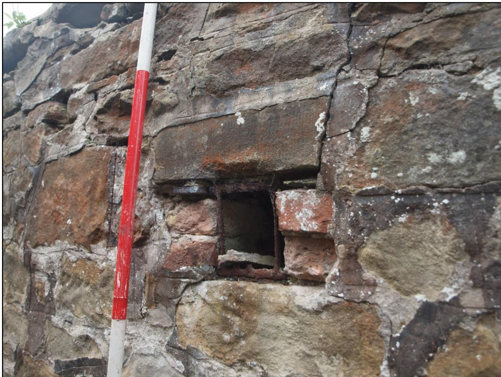
Plate 16: Hole within northeast elevation
