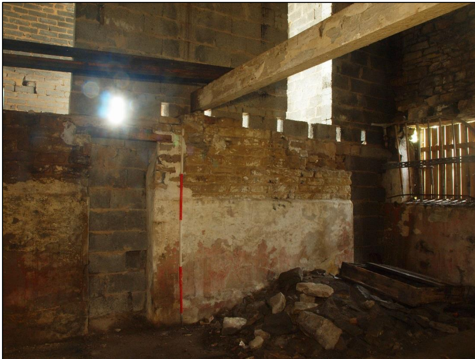
Plate 48: Blocked doorways in south wall
