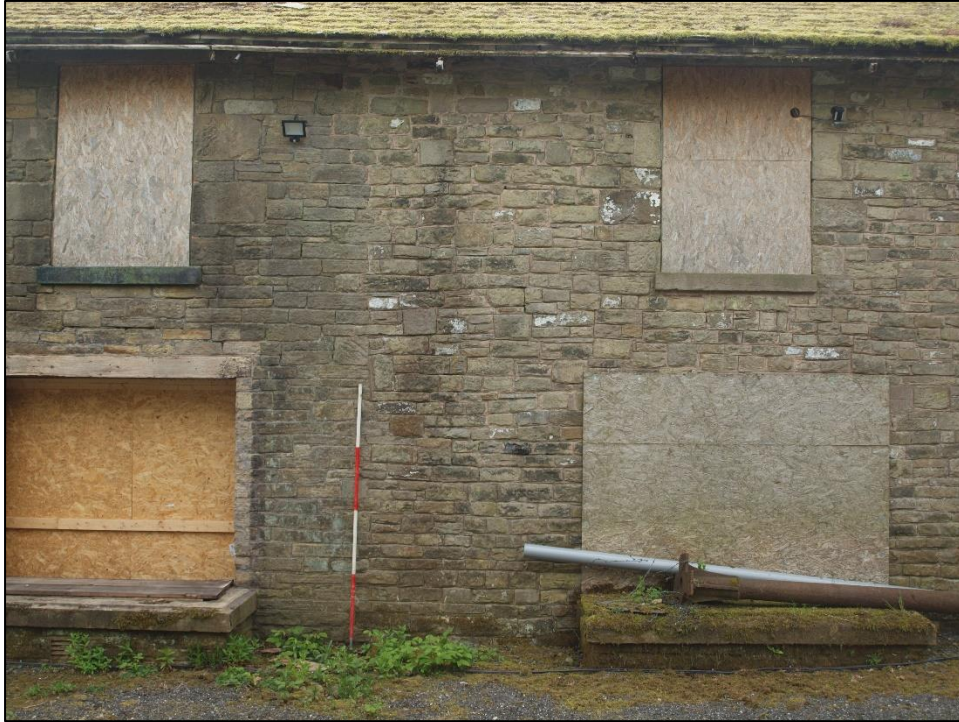
Plate 23: East end showing rough joint
