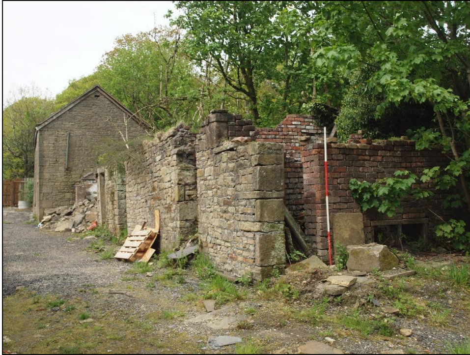
Plate 87: Southeast corner of outbuilding showing doorway in southern end of east elevation
