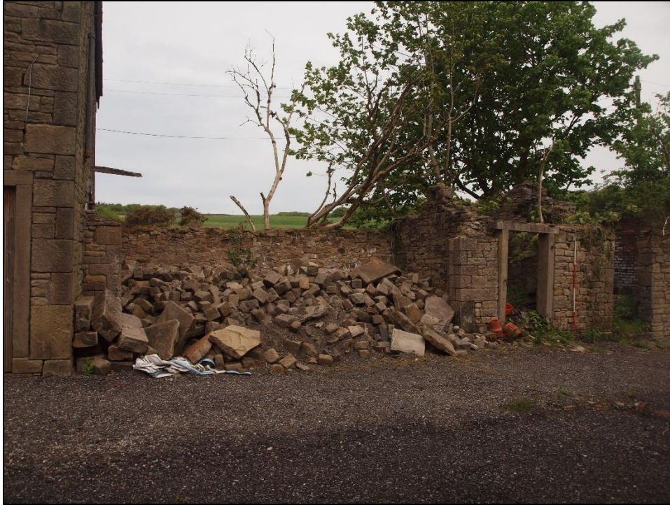
Plate 77: Collapsed outbuilding to east of barn
