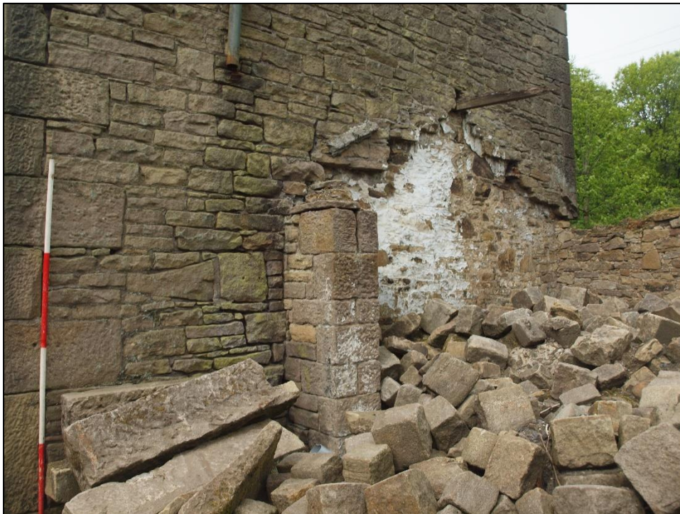
Plate 78: Interior of first unit showing wall scar
