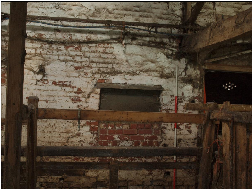
Plate 44: Blocked doorway to bay 3
