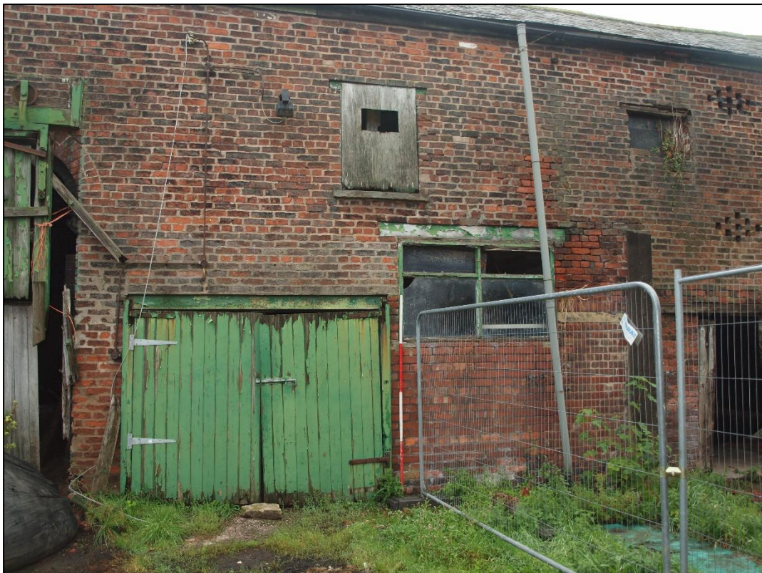
Plate 6: Doorway to bay 3 with inserted window above and blocked doorway to right
