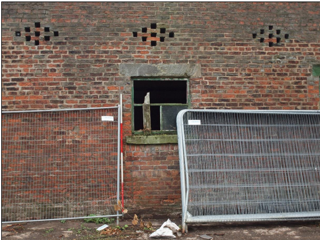
Plate 14: Blocked doorway to centre
