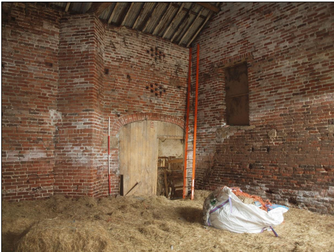
Plate 36: Threshing barn floor showing barn door to lean-to and high doorway to first floor
