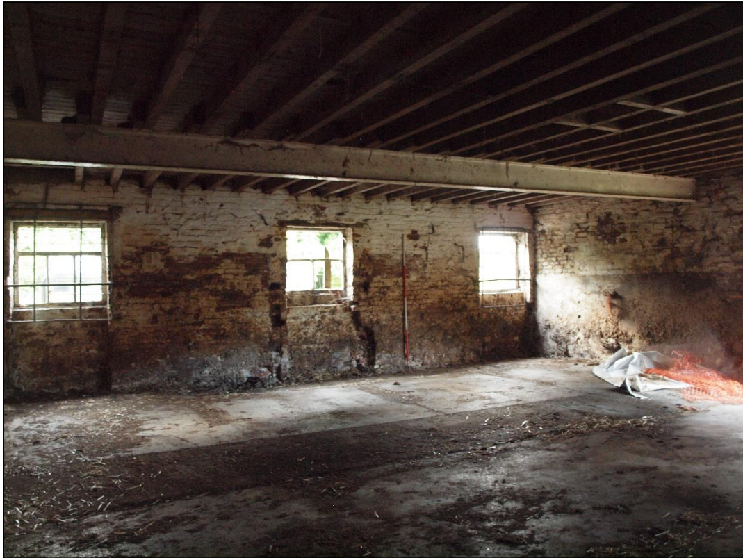
Plate 31: Blocked doorways in east gable
