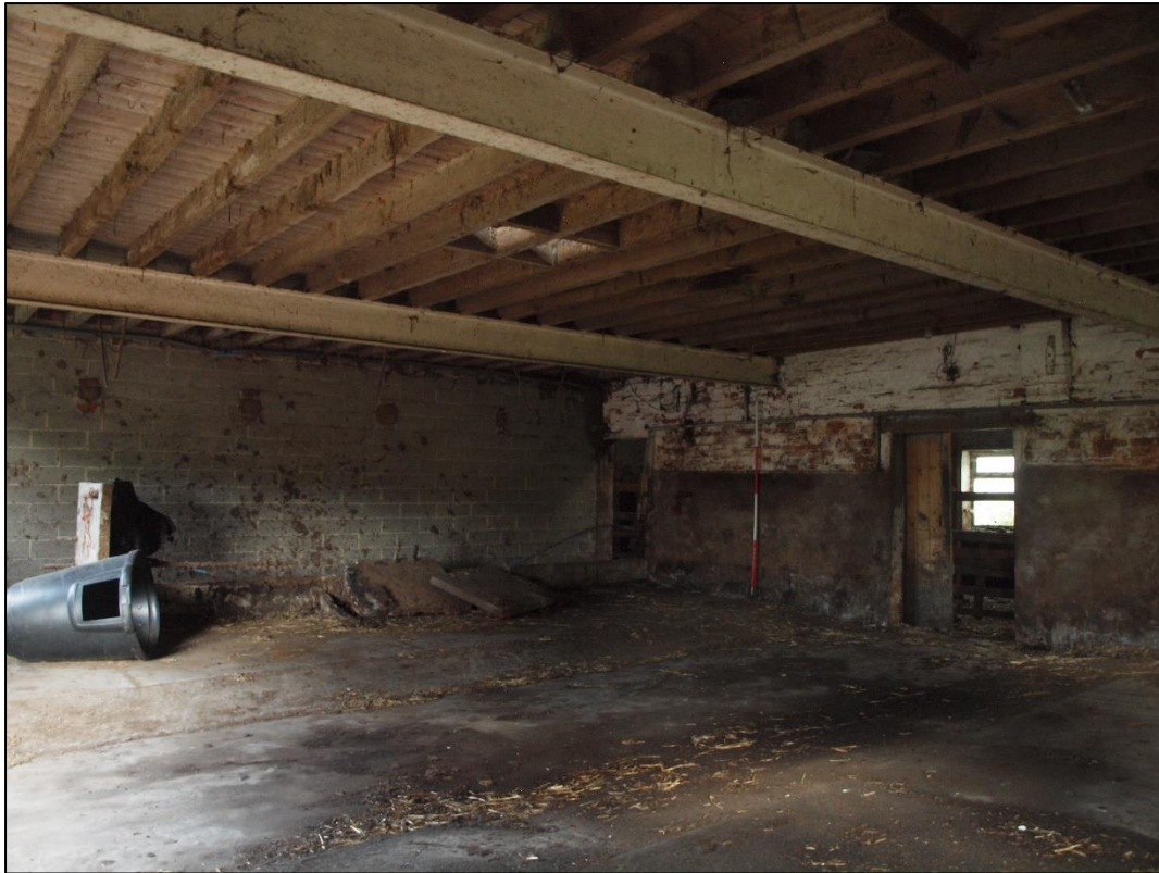
Plate 29: Interior of main barn, bays 4 – 5 showing inserted steel beams and concrete block wall
