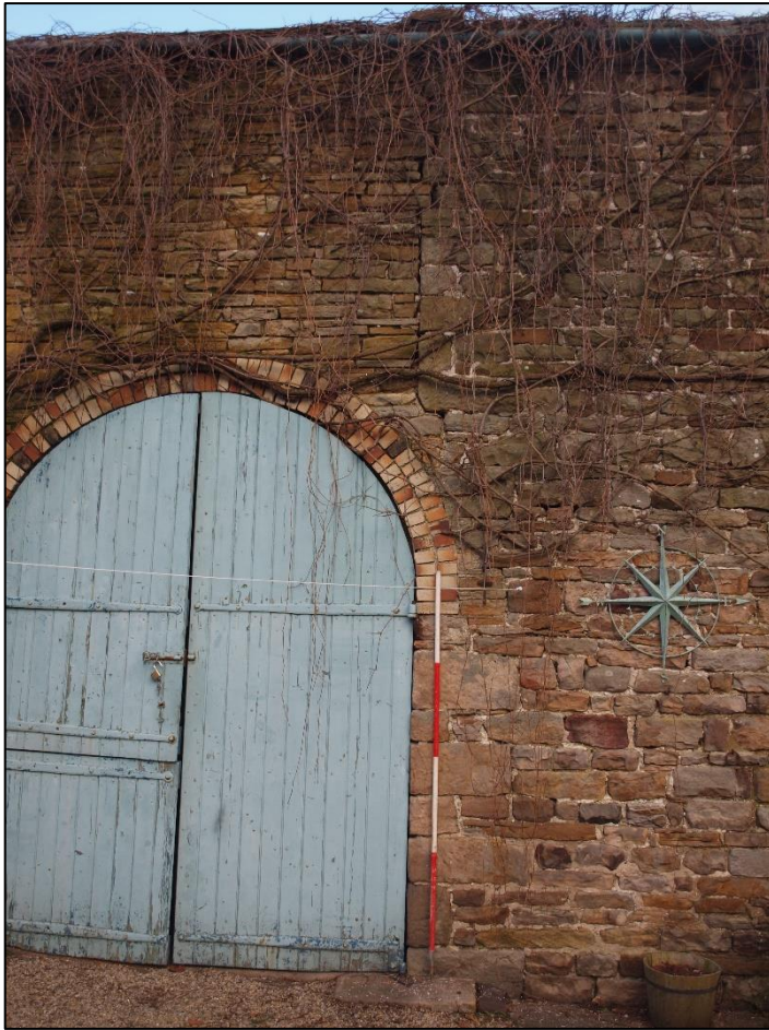
Plate 9: As above showing straight joint at first floor level looking north
