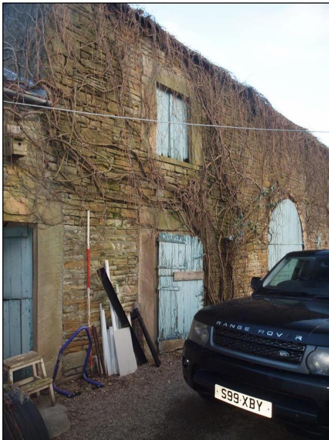
Plate 4: General shot of western end of south elevation showing bays 2 - 5 looking northeast
