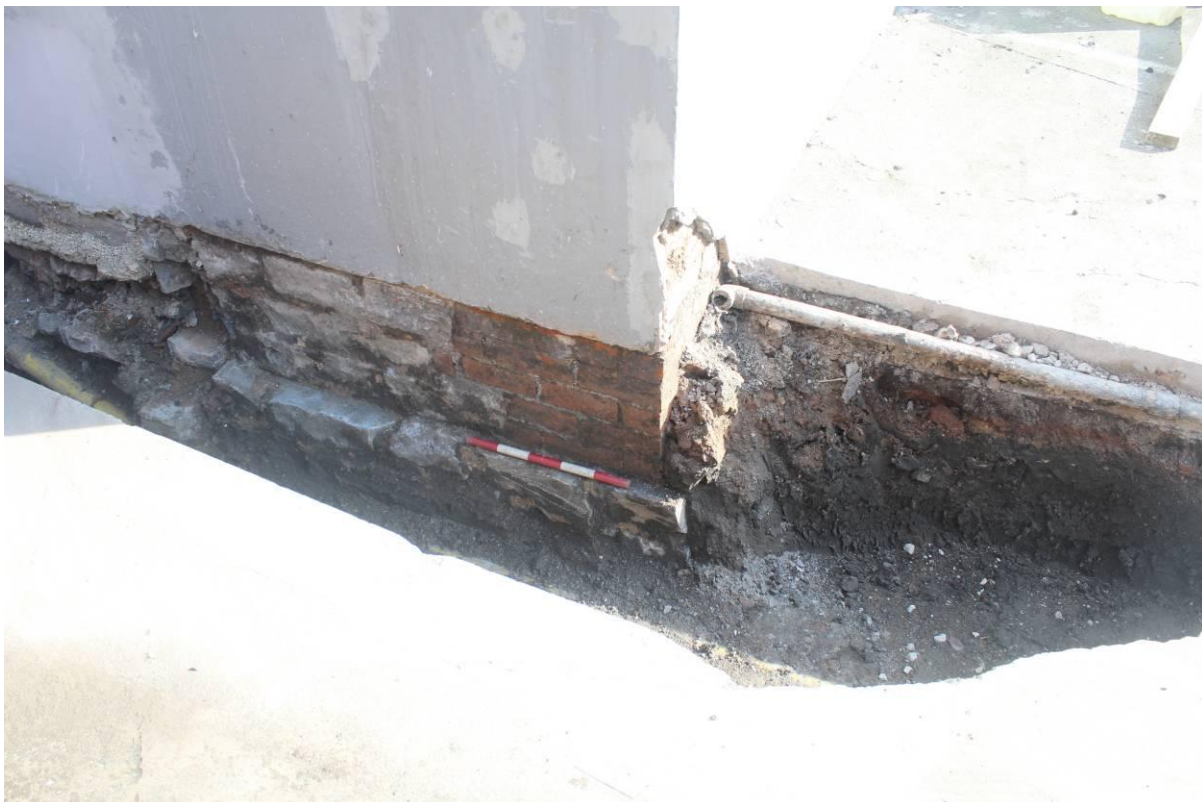
Fig. 6 Southwestern corner of St Nicholas House showing brick and stone foundation, looking northeast; scale 0.5m
