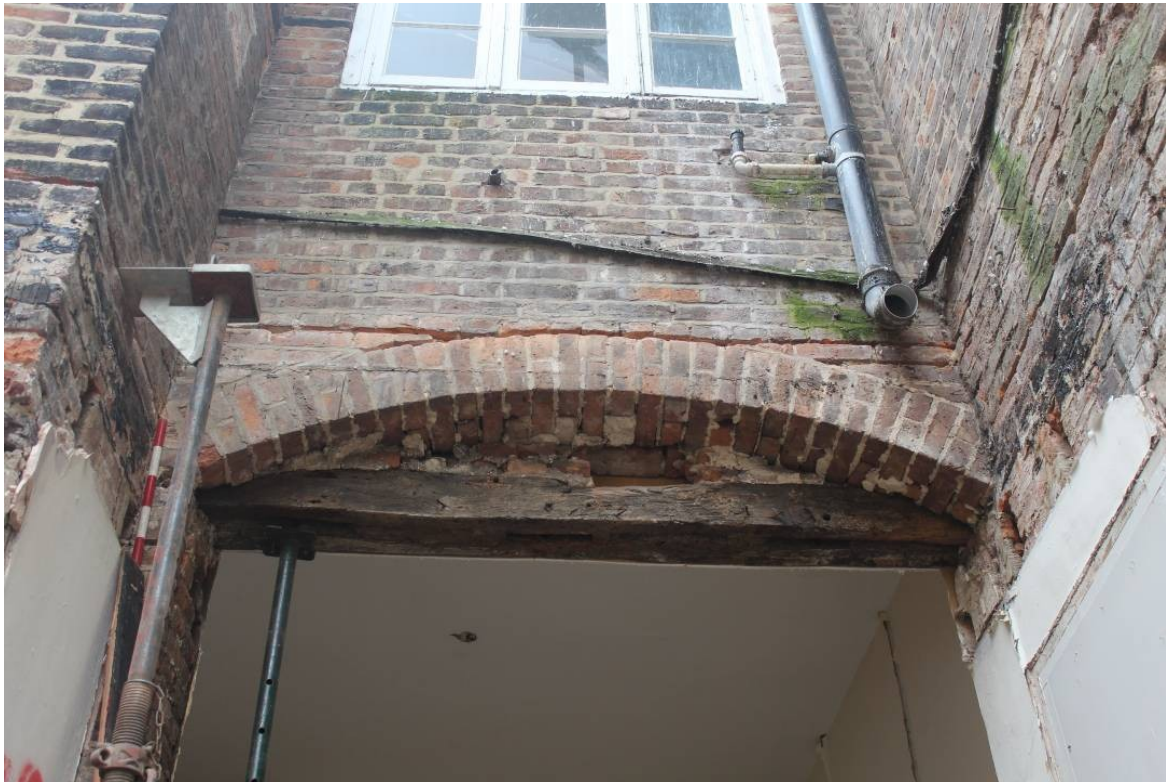
Fig. 26 Brick arch backed up by a reused oak timber with mortices; looking south, scale 0.5m
