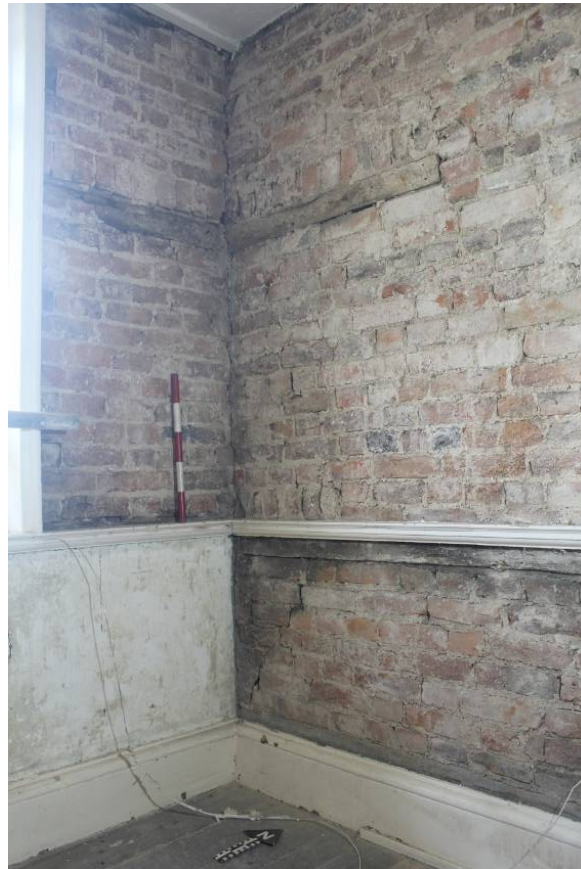
Fig. 24 Junction of western and northern walls of Monument House, first floor, showing bond timbers within brickwork, and butt joints between the walls, looking northwest, 0.5m scale
