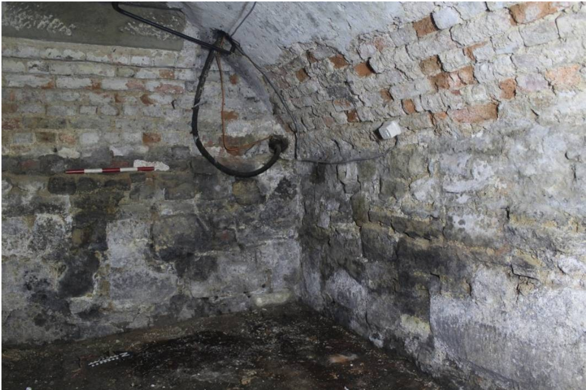
Fig. 16 West and north walls of Monument House basement, showing masonry basement walls with brick barrel vaults; looking northwest, scale 0.5m
