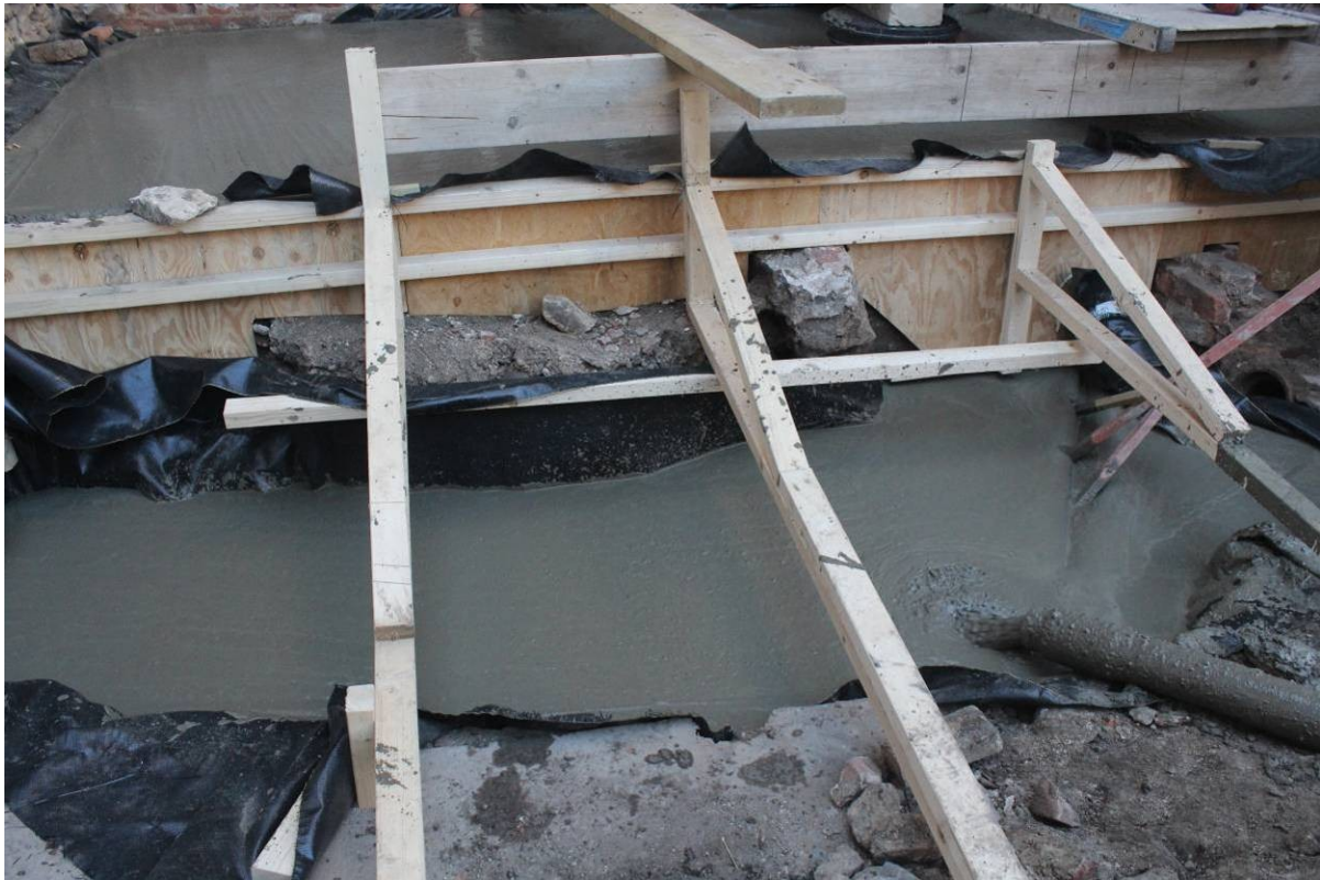
Fig. 30 Pumping of aerated foam concrete into the northern foundation trench, with Terram separation to the surviving archaeological deposits
