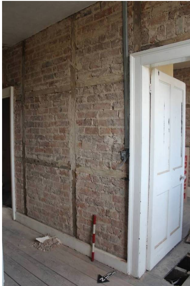
Fig. 22 Pegged timber studwork with mortared brick infill, second floor of Monument House, looking southeast, 0.5m scale.
