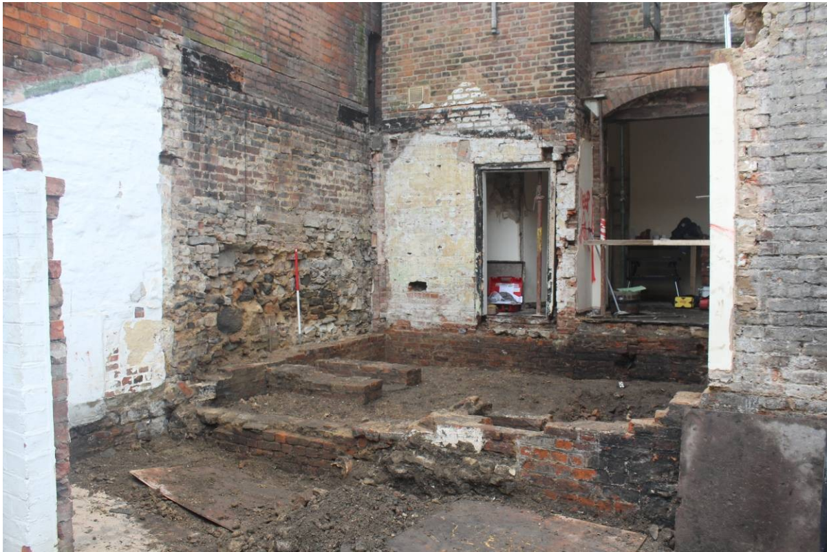
Fig. 12 Courtyard area looking southeast, with brick wall [11] forming northern boundary of courtyard, brick wall [2] forming the east wall and parallel walls [24] and [25]; note gable roof scar on north wall of Monument House and poorly built lower section of Community House extension [3]; scale 1m
