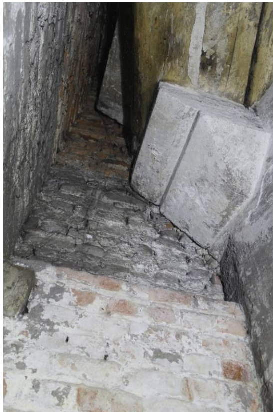
Fig.17 Masonry north wall, projecting corbel and beams of St Mary's Gate, with abutting brickwork of Monument House built around the existing masonry; looking east upwards from the doorway in north side of St Mary's Gate
