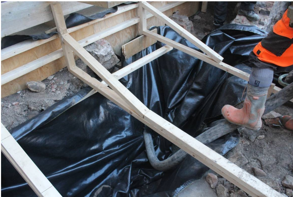
Fig. 29 Use of pumped aerated foam concrete to fill the culvert, the concrete is pumped along a pipe inserted through an existing hole in the culvert to fill the void and support the roof of the culvert.
