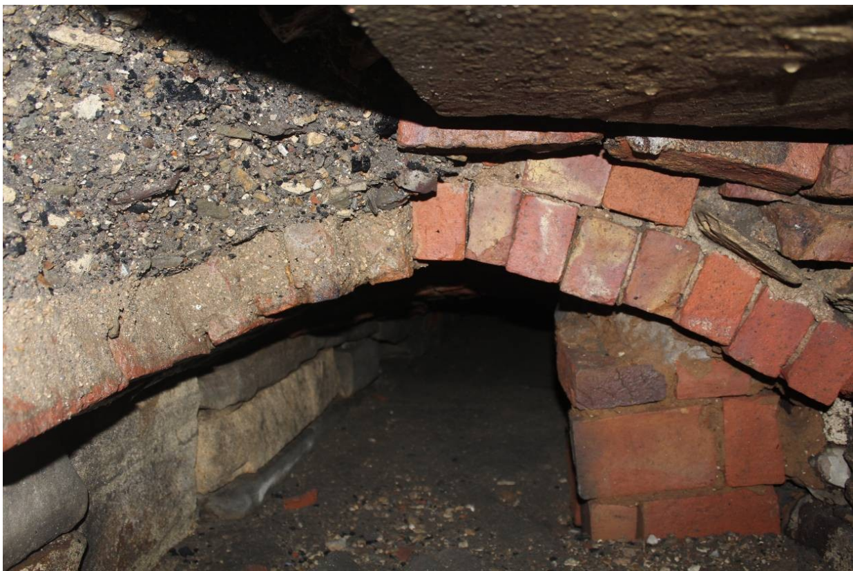
Fig. 7 View looking along masonry culvert [34] showing brick arched roof [31] with brick support; no scale
