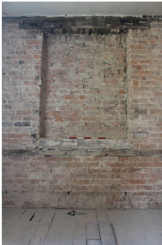
Fig.27 Blocked window in east wall of Monument House, second floor, showing mortar and lathe and plaster demonstrating the window was originally open; looking north, scale 0.5m
