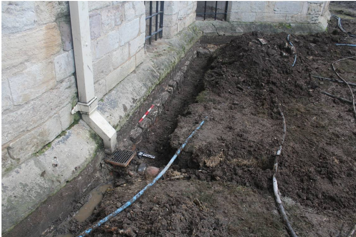
Fig. 5 View looking east along south wall of South ambulatory showing curve of foundation [4] compared to straight line of superstructure; 0.5m scale
