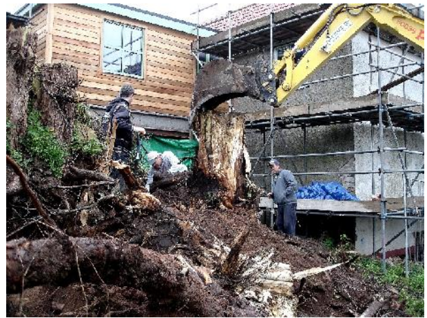
Plate 10 – Removal of tree stumps from part of former pub garden revetment. View to south-east.
