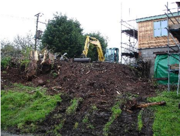
Plate 11 – Clearing and pulling back on top of the former garden revetment at the north-west side of the site. View to east-north-east from Camp Road.
