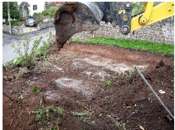
Plate 12 – Clearance work with mechanical excavator in the area behind (ie to the east of) the former revetment wall, showing shallow concrete base of former wooden shed. Camp Road can be seen top left. View to north-west.
