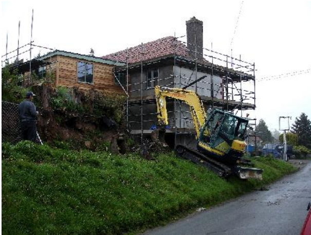
Plate 9 – Initial clearance of the bank fronting onto Camp Road prior to commencement of groundworks at the north-western corner of the site. The section which had been examined during the evaluation phase, following removal of the revetment wall on the western side of the pub garden, can be seen towards centre left. View to south-east.
