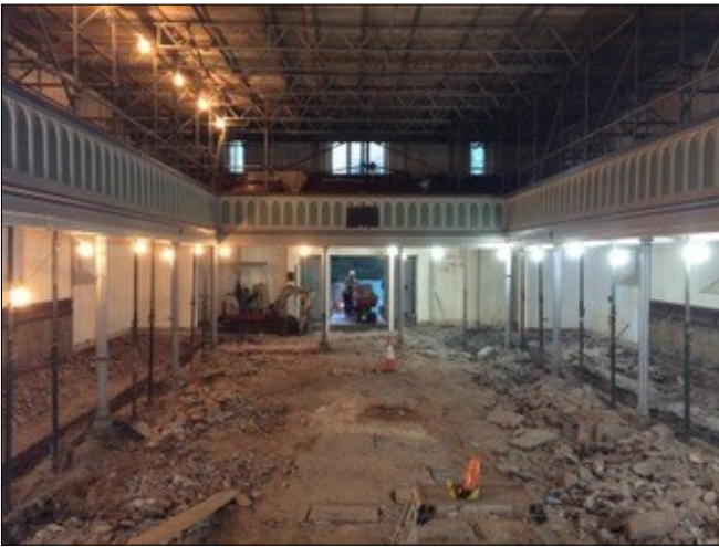
Plate 1: Work to remove the floor within the nave, view west (photo courtesy of M. Nichols).
