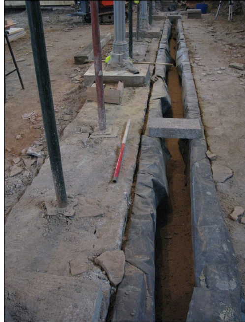
Plate 8: New services trench, parallel to structural support wall, within the south gallery of the nave, view east.
