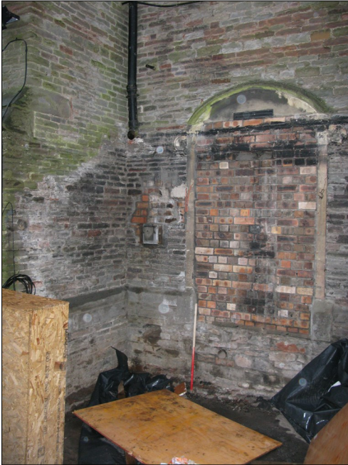
Plate 7: The blocked south entrance to the Church. A lean too structure which contained a gas boiler has been removed, but the scar is visible on the stone work.
