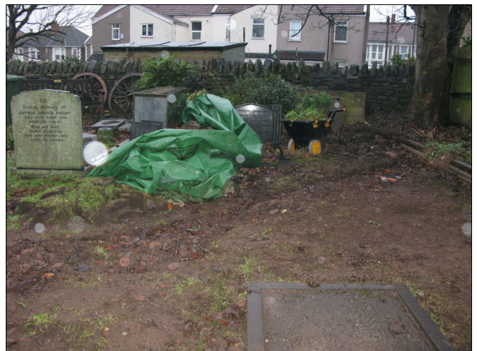
Plate 6: Back-filled services trench, diagonally across shot, to wards mains connections in North Street.
