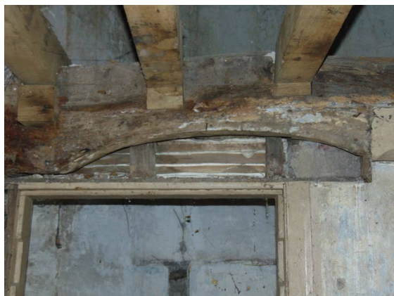
Plate 60: Detail of lintel over former stairway entrance adjacent to the fireplace in room G10.
