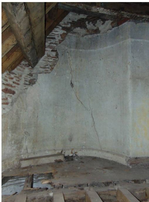
Plate 61: View of curved wall of former staircase in first floor room F5.
