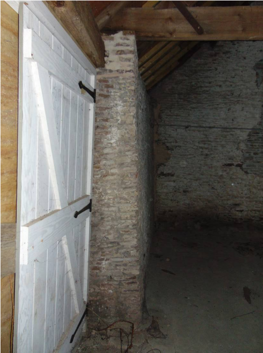
Plate 63: Detail of splayed base in Barn C. Looking north at western doorway.
