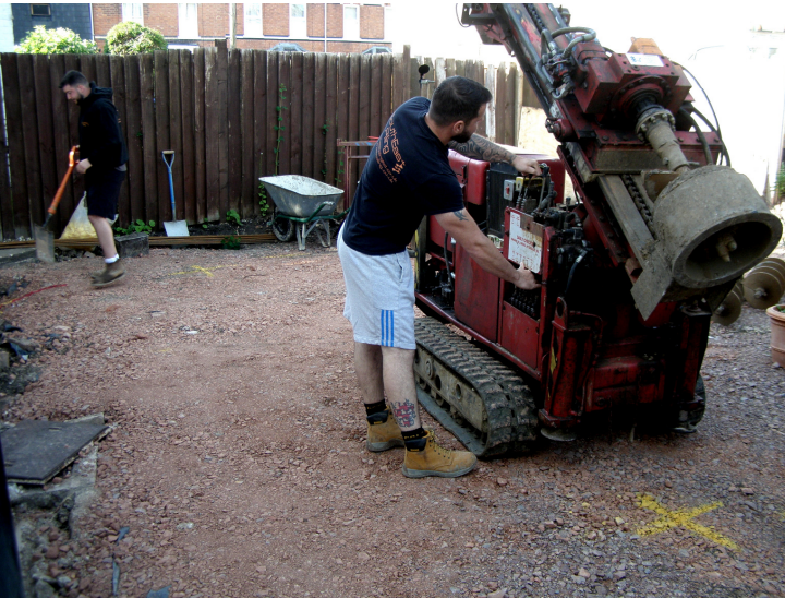
1. Preparing the rig for operation. The yellow cross at bottom right marks the first, and deepest of the pile holes to be drilled, and is the north-westernmost of the group as marked on Figure 3 . View to south-west from the north-eastern side of the site.
