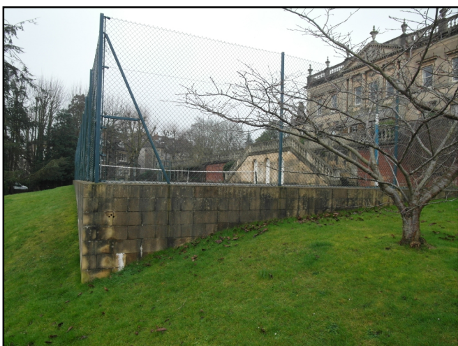
4. Revetment walls containing the upper tennis court, showing the degree of cutting and filling that was required to create a level playing surface. View to west.
