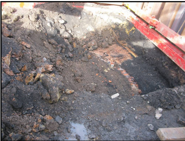
3. Trench 1 during excavation, from south-east, showing Cut [108] with Fill (107) to right of frame, and northern edge of Shaft (104).
