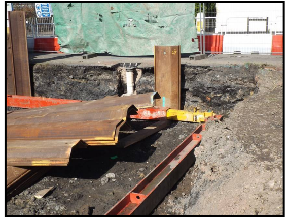
2. Trench 1 during insertion of sheet piles, showing south-facing section, to a depth of 1.2m.
