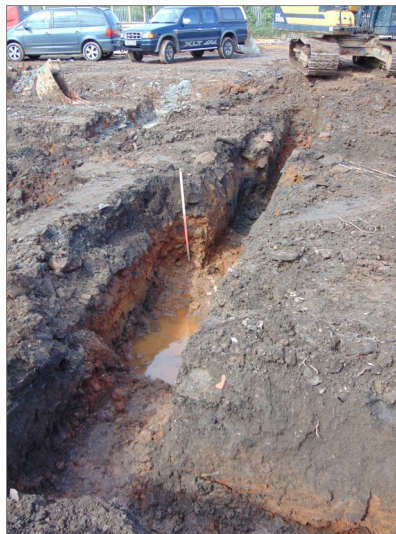
Plate 25 Foundation trench for House 2, just clips the edge of the building recorded in House Plot 1 excavation. View south west.
