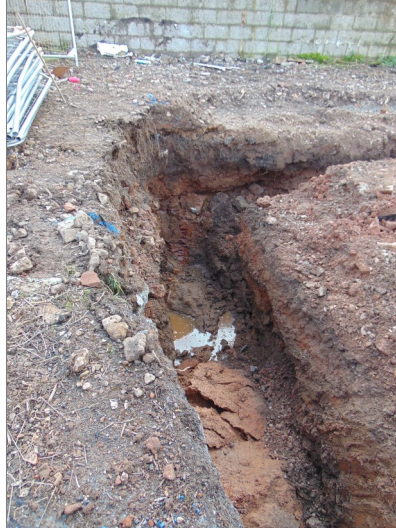
Plate 22 Foundation trench for house 3, unstable deposits collapsing into the open trenches as they were dug.
