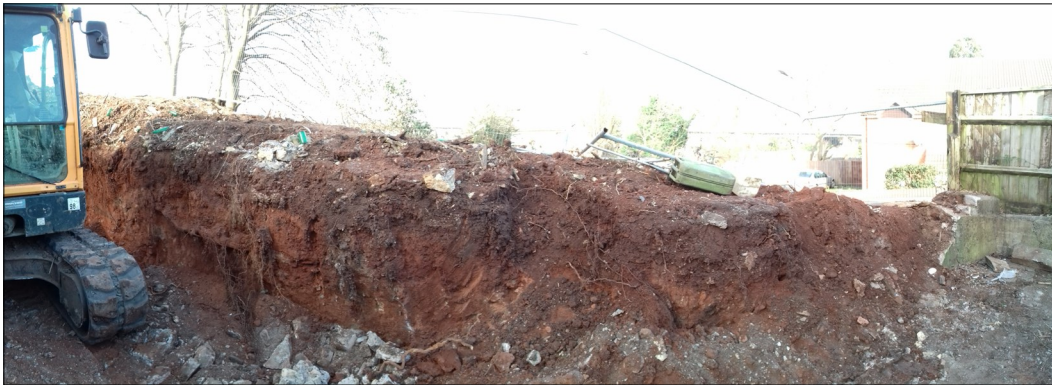
Plate 2: Panorama of south facing section through the hillside on removal of original garage.
