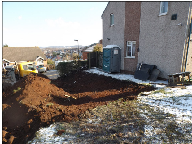
Plate 5: Topsoil strip of development footprint, looking east towards the side of number 75.
