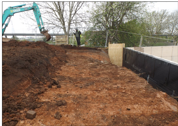
Plate 6: Topsoil stripping to the rear of new garages, exposing sterile natural ground.
