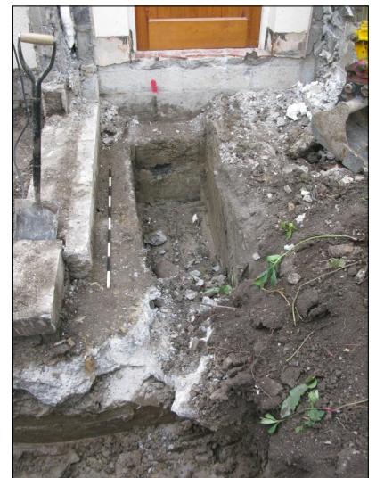
Plate 5 Photo shows the exposed concrete footings of the entrance porch which was recently removed to make way for the new extension.
