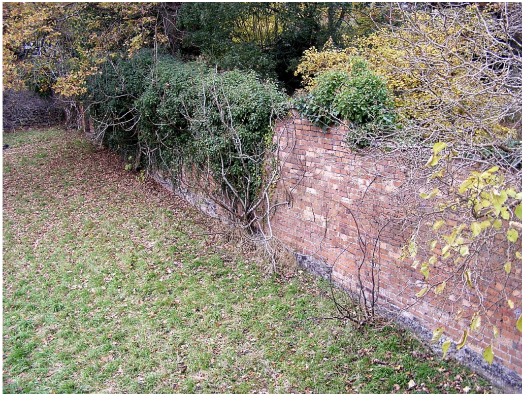
5. The main garden wall marking the north-western boundary of the stable annex site at Burwalls running north-east/south-west, it's south-western end joining with the boundary wall onto Burwalls road. Although for the most part now constructed of brick, it rests on a stone-built base, just visible in this image, which almost certainly represents a remnant of the original early 19th century kitchen garden wall belonging to Keeper's Cottage, now gone but originally occupying a site on the western side of Burwalls Road. This may well represent, therefore, the earliest built structure on the entire site. View to north-west from an elevated position in one of the modern annex buildings.
