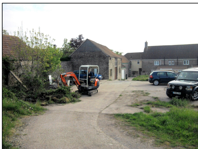
a) General view of study site from west, before excavation, showing concrete yard surface, barns in centre rear of frame and ground sloping down to east.
