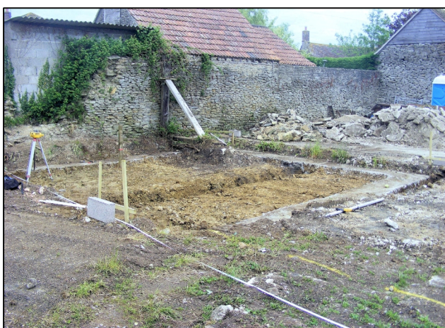
c) Area A from south-west, after removal of concrete, showing natural orange clay (102) and boundary wall to north.
