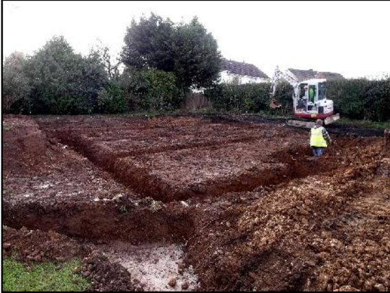
12. House 3 foundation trenches completed. View to west. In the foreground, concrete has been poured into the foundation trench for the south-eastern boundary wall (see Figure 3 ).
