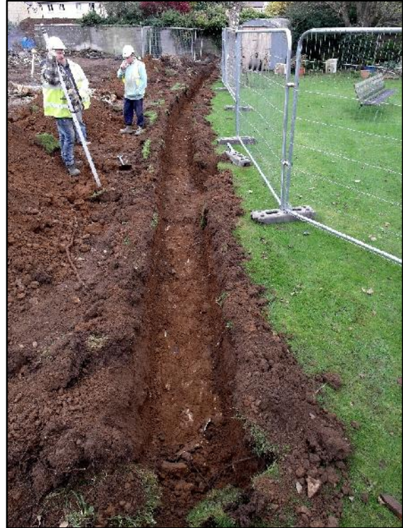
5. Foundation trench for new boundary wall on the south-eastern side of the site nearing completion (see Figure 3 ). View to north-east from close to the south-western end of the trench.
