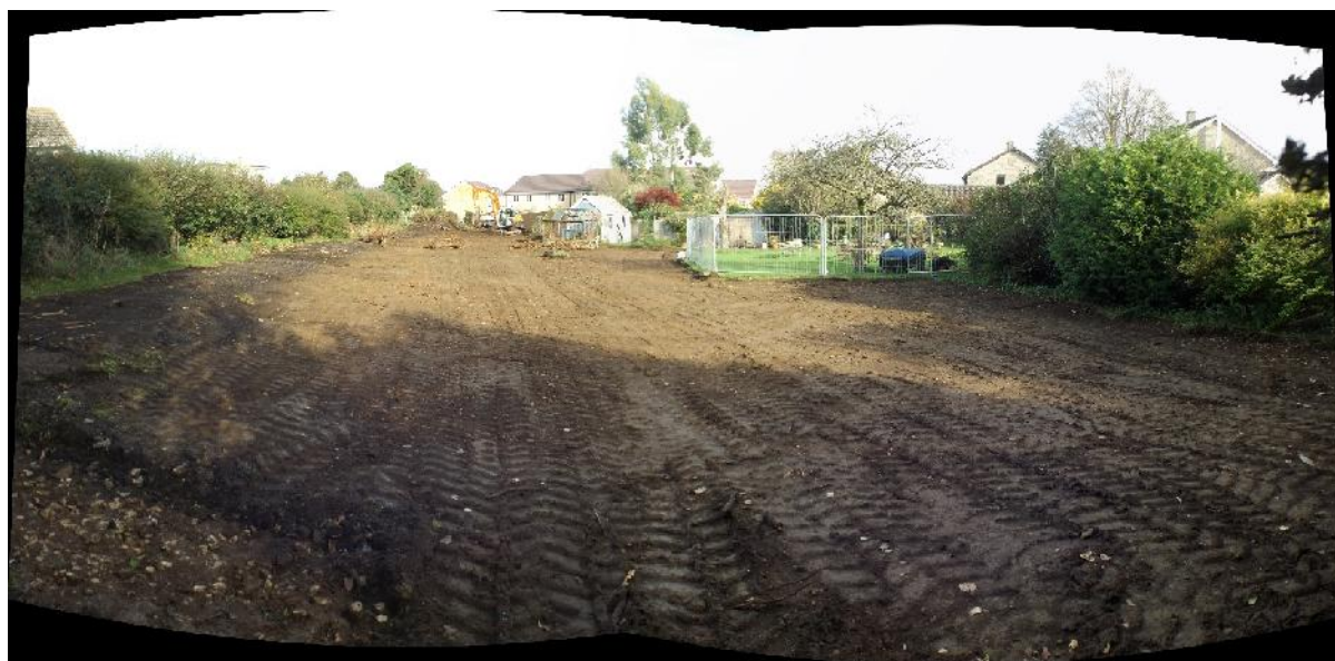
3. Composite panoramic image of the main site, with topsoil stripping complete. The view is from close to the south-west extremity of the site, and pans round from the north-west (l/h side of frame) to north-east (r/h side). Note, on the l/h side, the line of the probably early 20 th century cinder trackway running north-east/south-west, along the site's north-western boundary. It would have originally run underneath the boundary hedge on that side.
