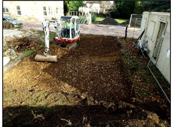
13. Completion of topsoil stripping in the former garden of one of the two pre-existing houses outside the development boundary, at the entrance of the new estate just off Wells Road. The work was carried out to install new driveways in front of both houses, and the image shows that for the westernmost house, shown on Figure 3 and known as Towerhurst . In the background, behind the excavator, the easternmost of the two houses can just be seen, together with the spoilheaps from the stripping of its own garden.
