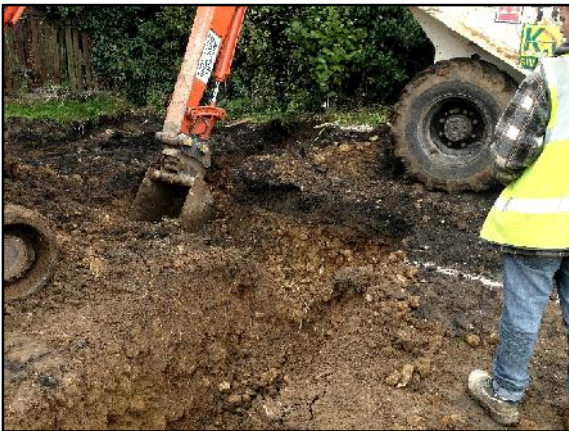
10. Image taken at the point where the south-eastern wall of the garage joins onto the north-western wall of House 3 (see Figure 3 ). View to west. Note the depth of the cinder trackway at this point, and the way that it has almost entirely truncated the subsoil layer in this area, to sit almost directly on top of the heavily weathered natural Lias limestone and
