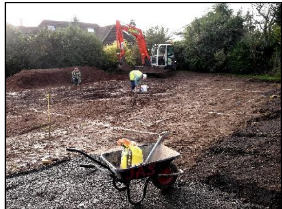
7. Marking out the trench lines for the foundations of House 3, at the extreme south-western end of the site. View to south.
