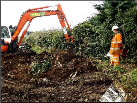
4. Using the machine to remove a large tree stump at the north-eastern end of the site, in the middle of the line of the new access road. View to south-west.
