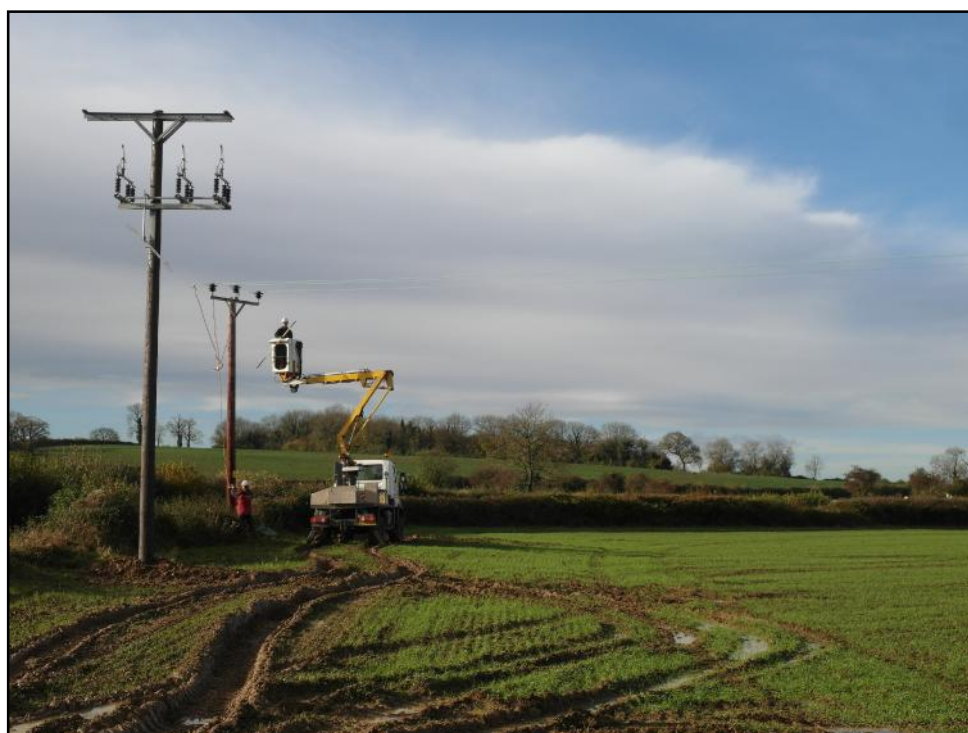
Frontispiece: Using a mobile elevator to isolate the power supply to the existing overhead cabling, prior to integrating the new poles and cabling into the network. View to west-south-west.
