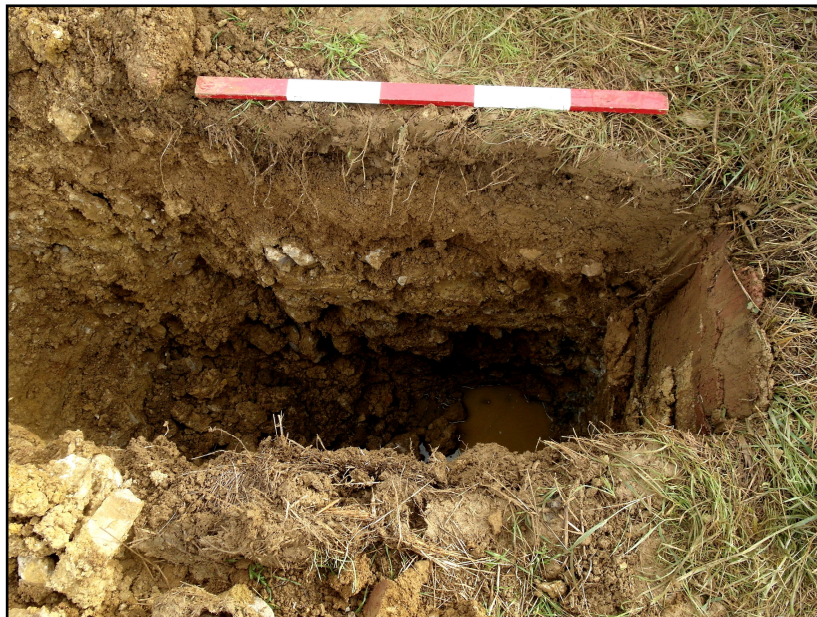
2. Hole 4, for the final, westernmost pole. West-facing section. Note the slope down from the northern (left-hand) end. Only the southern end, where the pole base itself will sit, is at full depth (1.8m). Scale: 1m.
