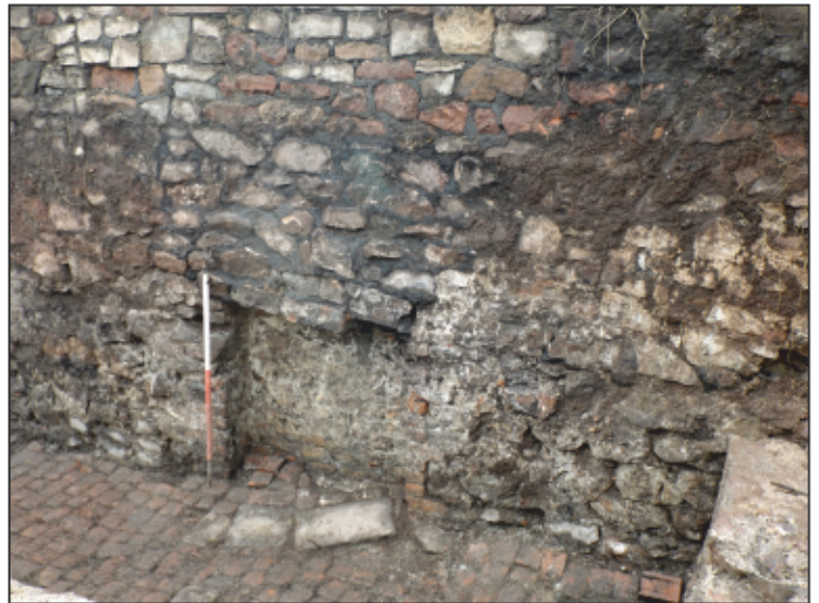
8. Feature (103), another blocked opening, possibly a doorway. Although the full blocking of this feature survives intact, it is also expressed on the external (southern) elevation of the main boundary wall (see Plate 10). Scale: 1m. View to south.
