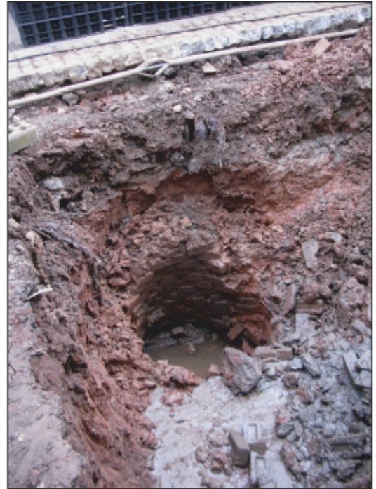
2. North-western side of the development, fronting onto the south-eastern side of Balfour Road, pit for soakaway, exposing brick-built well. The type of bricks used suggests machine manufacture and therefore relatively late construction, probably late 19th/early 20th century. Use of a scale was impossible due to the depth of the pit and the instability of the surrounding deposits, but the water seen at the bottom is at at least 2.5m below the cobbles on the south-eastern side of Balfour Road at the top of the image. View to north-west.
