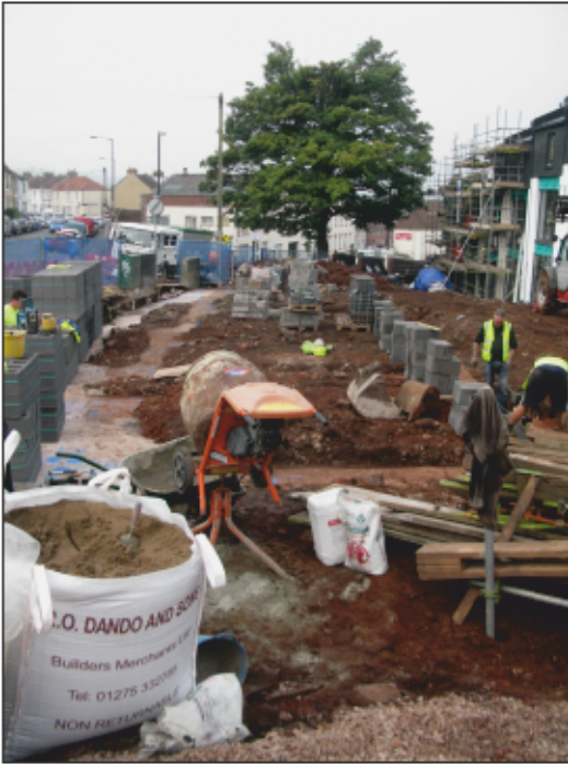
1. View to south-west from close to the north-eastern corner of the site. Footings of a small group of terrace houses fronting onto the north-western side of Luckwell Road, excavated and filled with concrete without monitoring.
