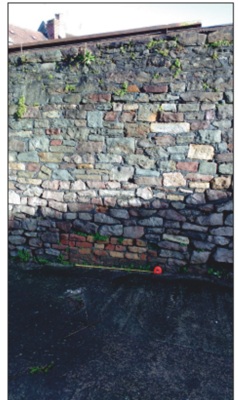
10. External (southern) elevation of main boundary wall, showing brick blocking of opening (103) in main boundary wall. See Plate 8. The tape in the foreground is extended to 1m for scale. View to north.
