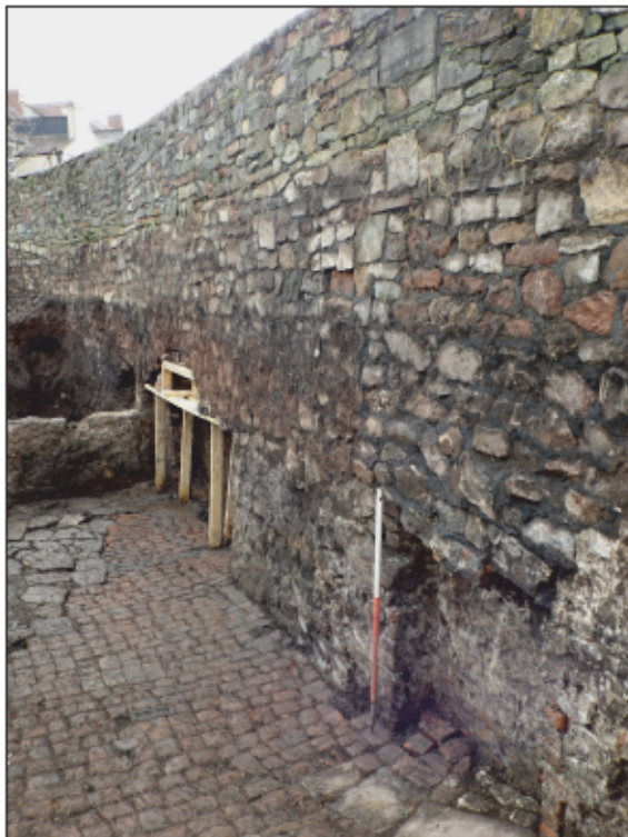
5. View of main boundary wall with (101) above white-washed elevation, and (104) below. Blocked opening (103) nearest to camera, (106) at further end with wooden bracing just inserted. Brick sett floor (105), with later flagstone repair (110), to bottom left. Note the 'tide mark' along the wall which indicates the depth of backfill removed to reveal these features. Scale: 1m. View to south-east.
