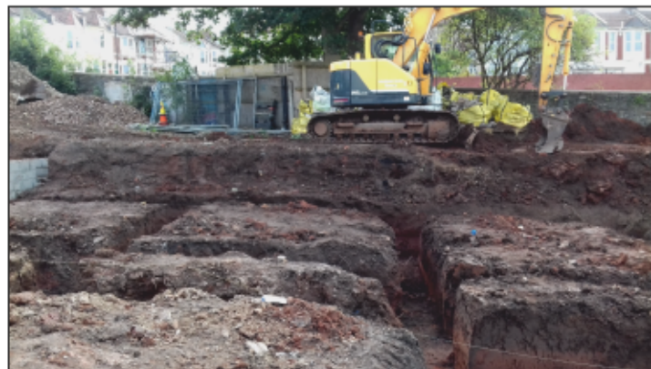
3. Footing trenches excavated in the central south-western part of the site, without monitoring. View to south-east. The main site gates in the top left part of the image open onto the north-western frontage of Luckwell Road.
