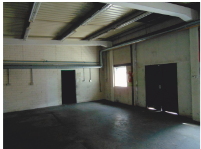
Plate 27: Looking north east at internal space of central range of the modern workshop building.
