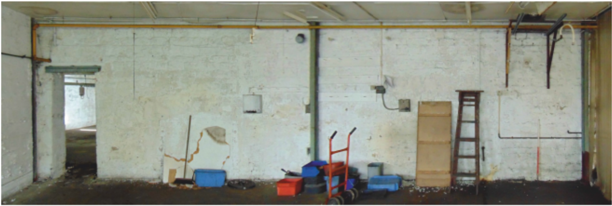
Plate 25: Looking north at 19th century wall reused as partition within the southern range of the modern workshop building (western end).
