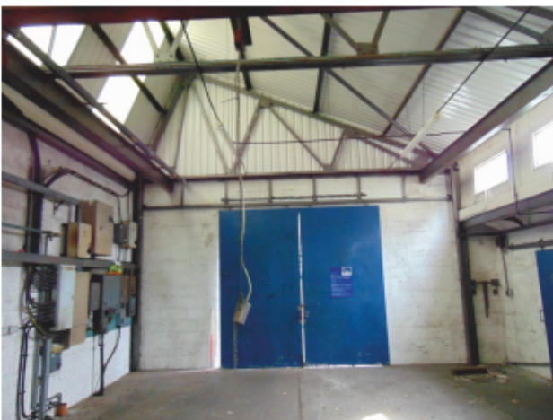
Plate 26: Looking east at west facing internal elevation of central range of the modern workshop building.
