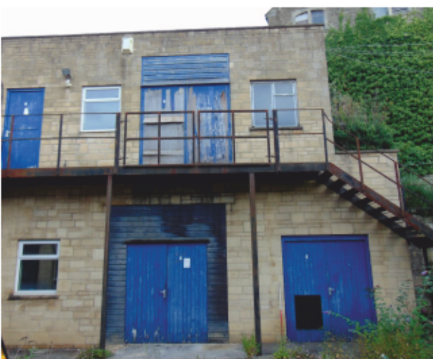
Plate 28: Looking north at south facing external elevation of northern range of the modern workshops.
