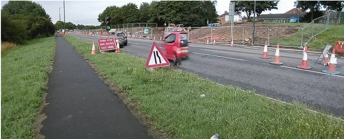
Plate 8. View along roadworks from opposite council offices (in the right-hand corner of the image), looking south-west
