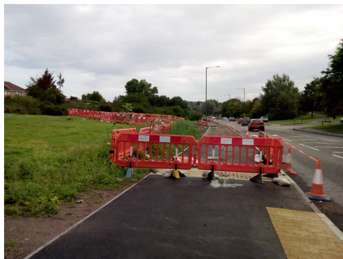
Plate 7. View of beginning of roadworks from opposite Two Acres Road, looking north-east
