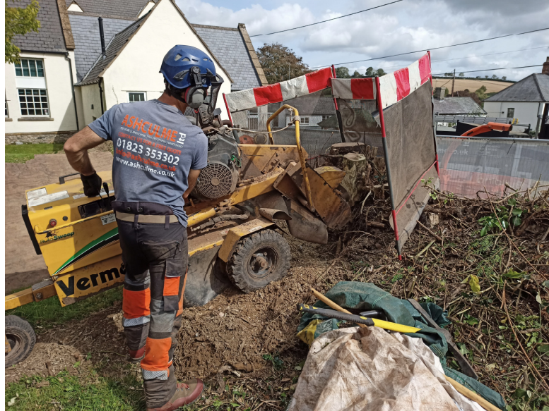
3. The larger remaining stumps were removed with a combination of a mechanical grinding machine (as here) and a mini-digger with a toothed bucket.
