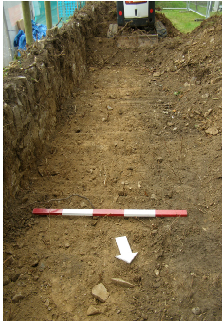
6. This work revealed what appeared to be a clear linear cut [103], in the darker churchyard material (105) to the right of the frame, (ie west), filled with a much lighter deposit (104) on the left (ie east). This is almost certainly a construction cut for the boundary wall (100), on the left of the frame. Scale: 1m.
