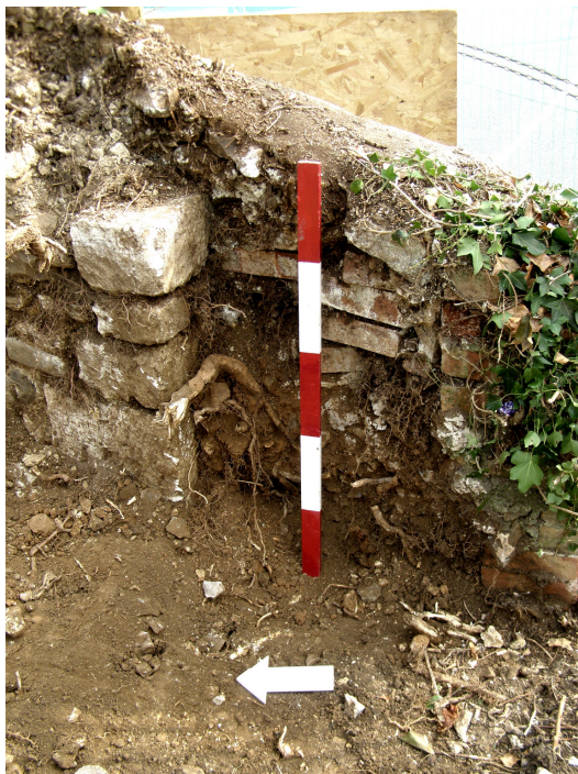
16. Probably modern brick extension at the southern end of masonry boundary wall (100). Note semi-ashlared stone blocks denoting the original southern end of the wall, probably acting as the northern jamb of an original gateway through it into the churchyard. Scale: 1m, north as indicated.
