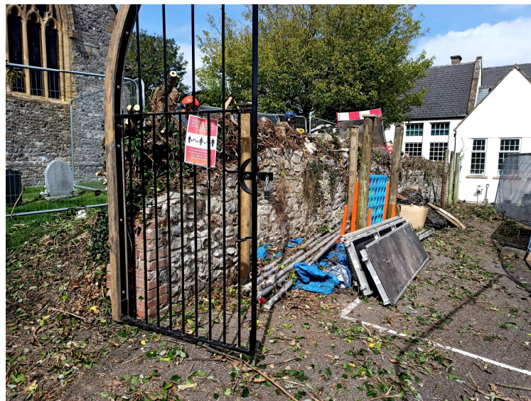
2. The main bulk of the hedgeline foliage removed, view to north-west from the eastern side of the boundary wall, in the school playground.
