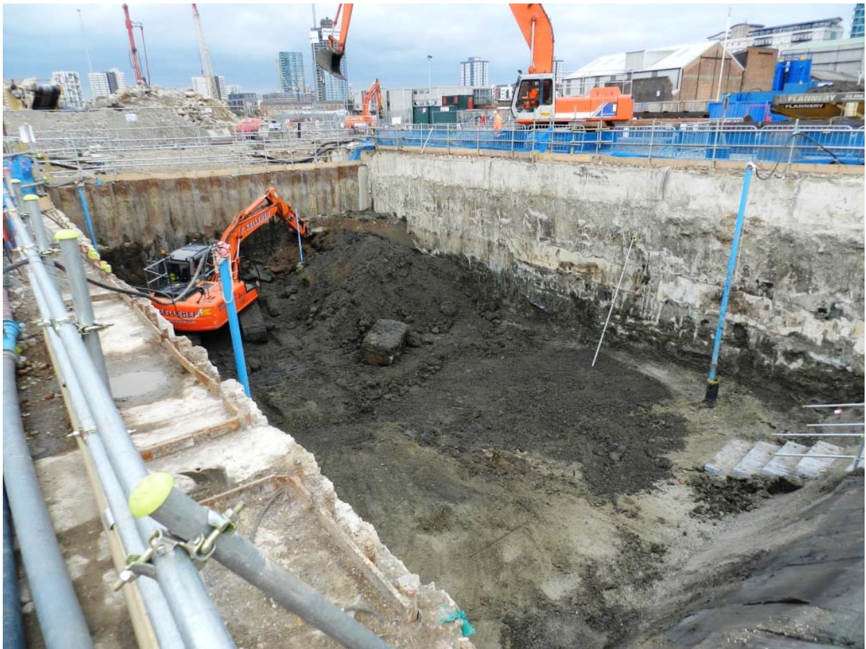
Photo 5 Cut and Cover Section 1 excavating through alluvium and into natural terrace gravels (last of concrete intrusions removed), looking east, 1st Feb 2011
