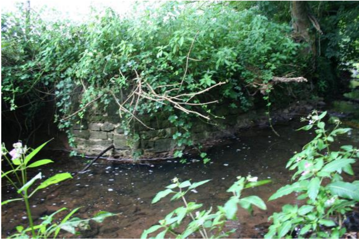
As you can see, there was a lot of vegetation to clear
