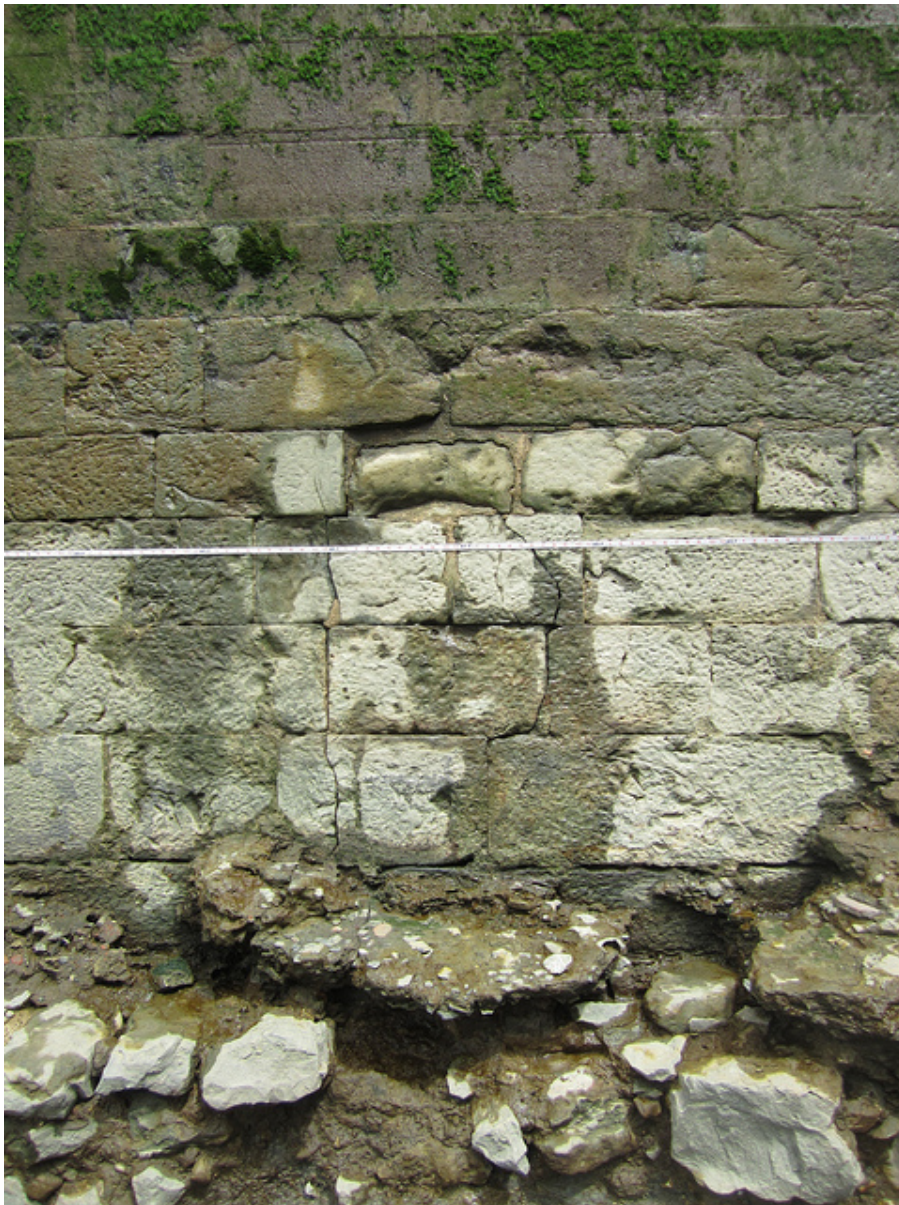
Cracks are starting to appear in the wall.
