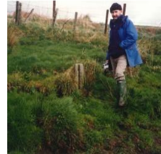
The slotted stone pillar of a sluice gate to control the flow of water over the meadow.
