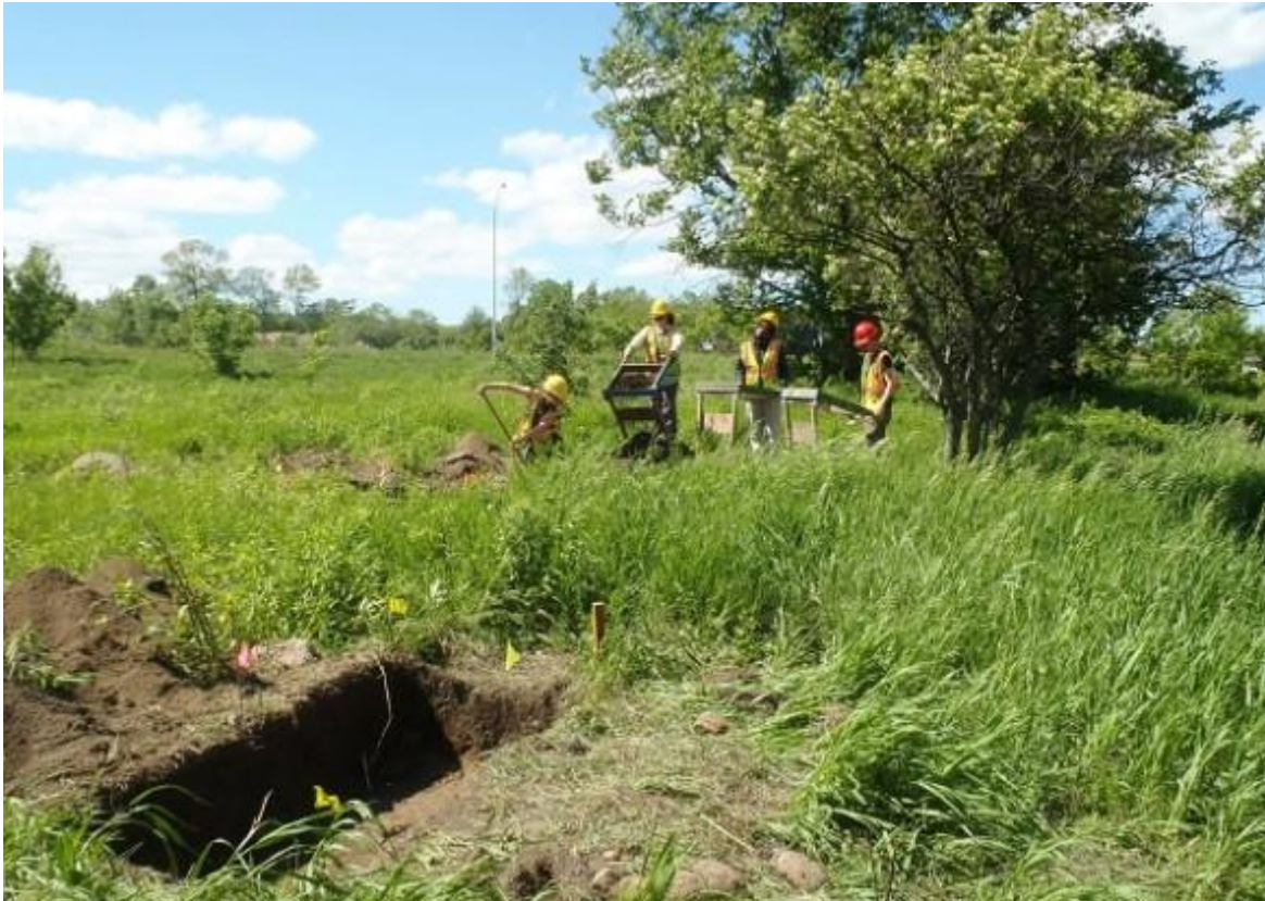
One of five crews working on the transportation project east of Toronto.
