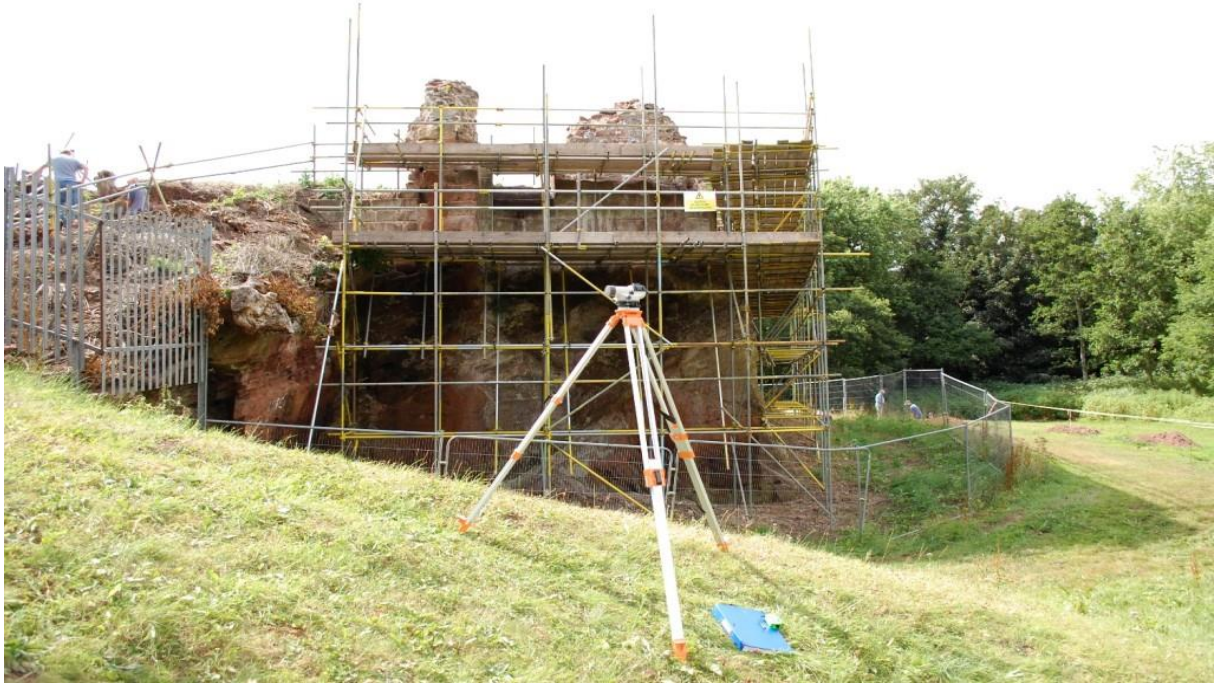
Excavation at Holt Castle – with Cadw, Northern Marches Cymru, Wrexham County Borough Council and Holt Local History Society all working in partnership.
