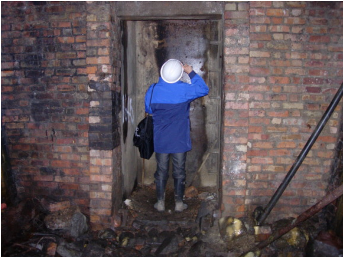
Blocked eastern end of the tunnel
