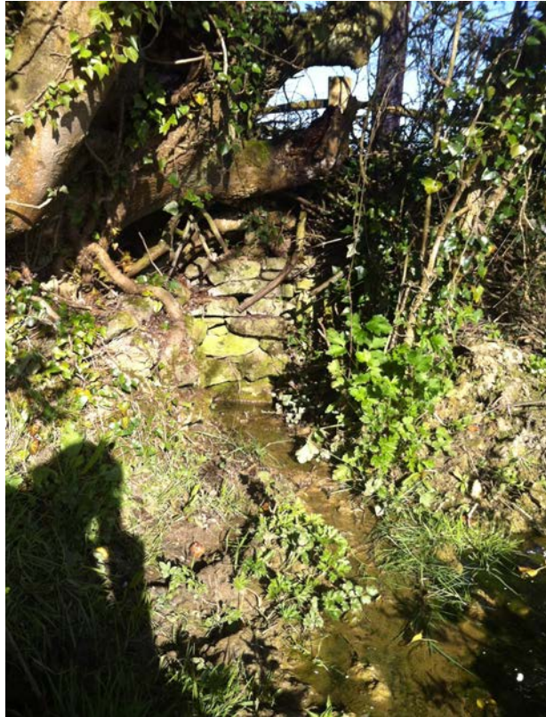
Appendix 9: Stone culvert at eastern end of Newlands ditch which feeds into north-south roadside ditch.
