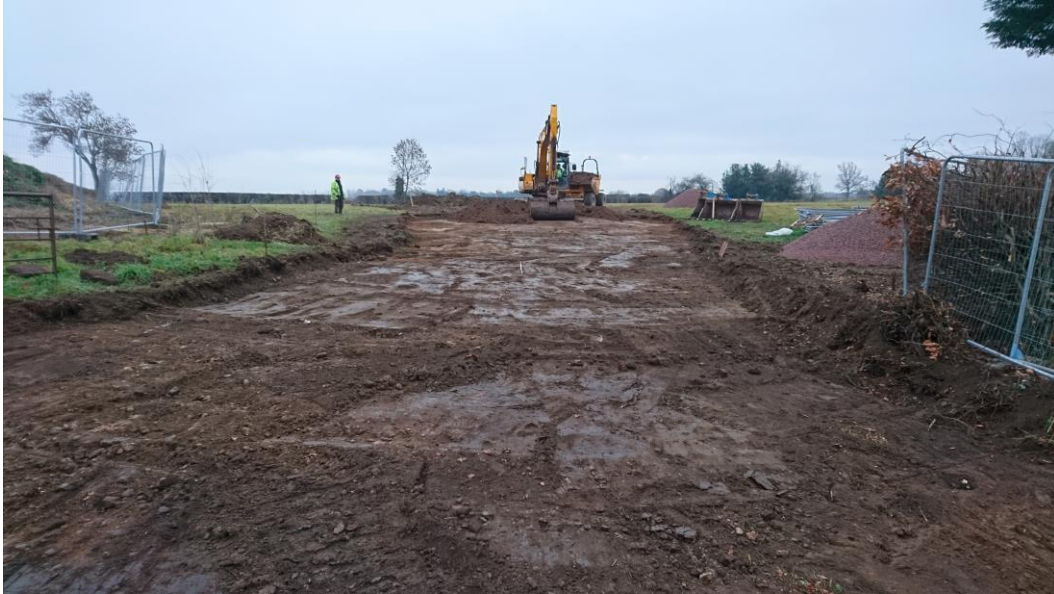
Plate 1: General view of construction area showing depth and extent of subsoil. 6 th December 2016. Looking south-east.
