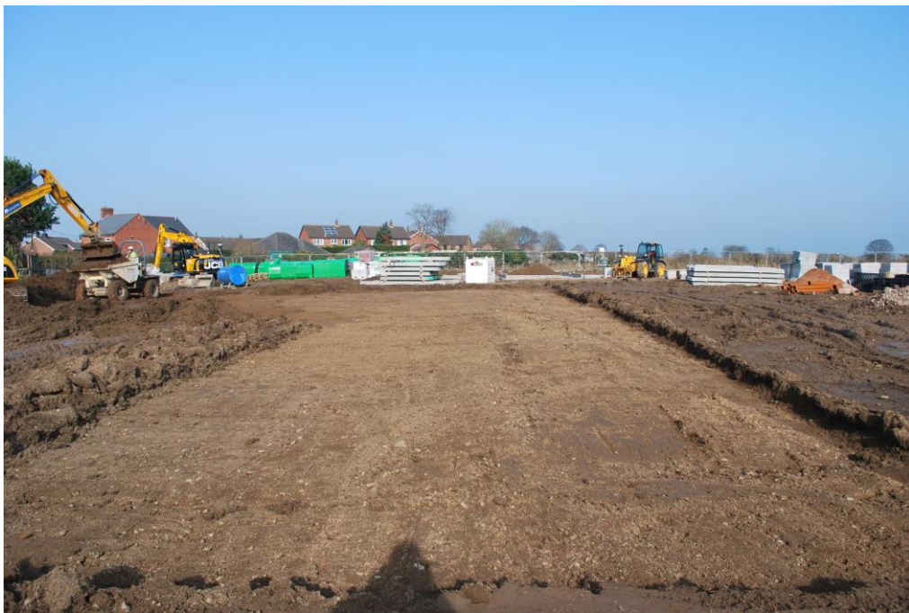
Plate 4: General view of construction area. Plough lines can be seen on the right of the stripped area. 13 th February 2017. Looking north.
