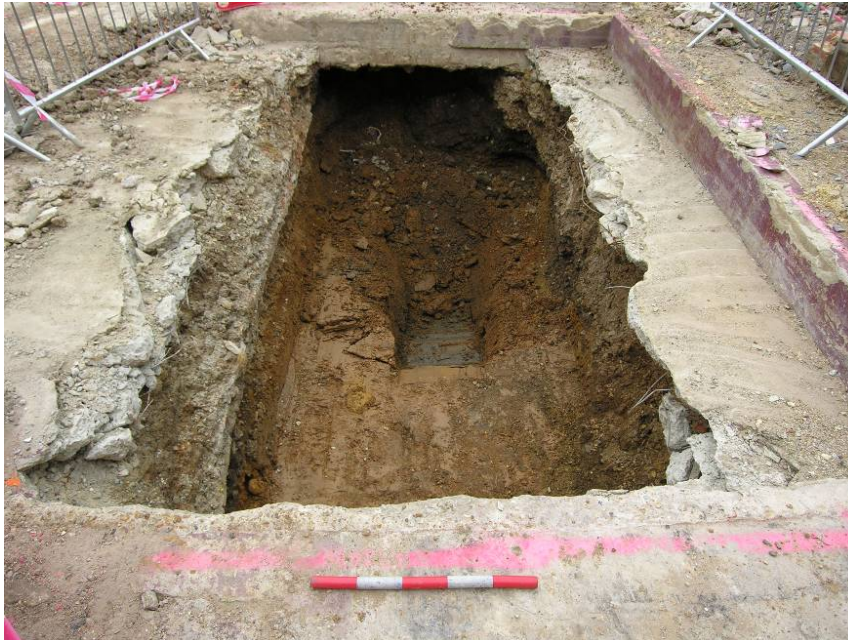
Photo 10, Trench 6, looking north. natural weathered London Clay (orange brown) overlying London Clay (in sondage, grey) at 11.90m OD (111.90m ATD).
